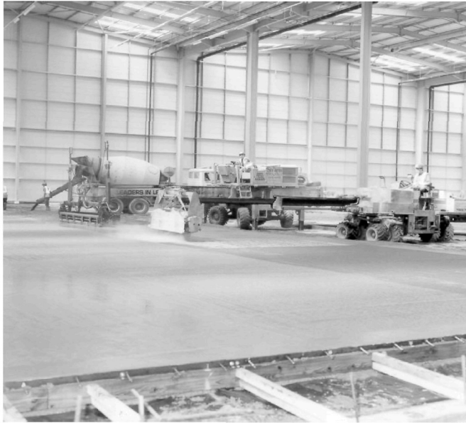
Figure 1 Highly mechanised floor slab construction using laser screed laser controlled spreader and alongside application of dry-shake finishing material
