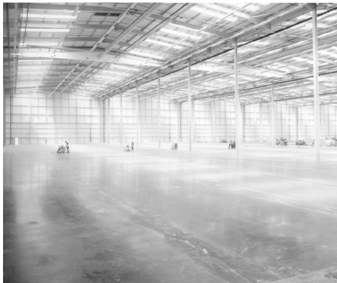
Figure 4 Sawing joints in a new warehouse floor with 10 m eaves height that will provide 30,000 sq m of storage capacity
