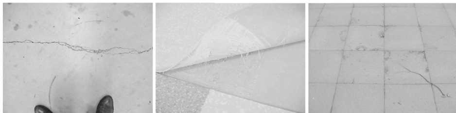
Cracks in concrete floors
