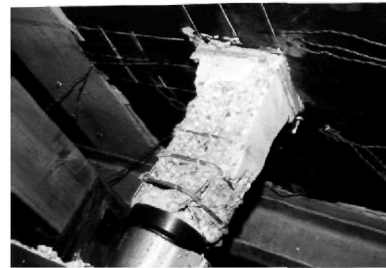
(b) S2: Failure of column by bursting
