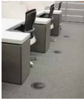
The grilles from this UFAD system are easily accessible so office workers can adjust their local environment.
