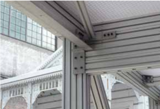
The Cellophane House (2008), designed by KieranTimberlake, can be disassembled, transported, and reassembled.
