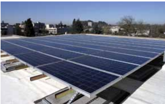
Conventional PV panels are mounted on top of buildings or nearby.
