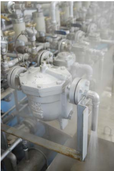
Figure 13.3. Before starting the steam trap management program, the plant should evaluate the current steam trap practices and determine whether the optimal technologies are being used. (Courtesy TLV Corporation. All rights reserved.)
