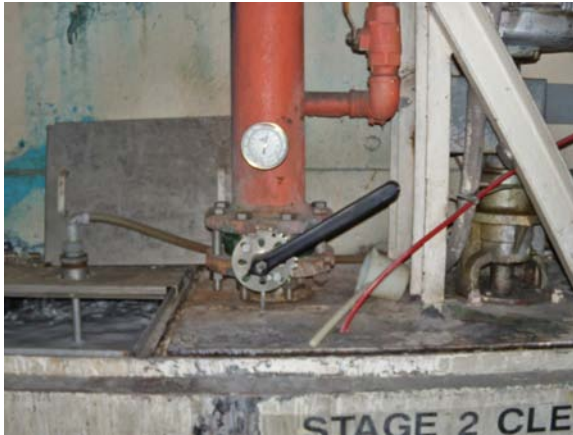
Figure 15.2. Throttled butterfly valve controlling flow on a parts washer.
