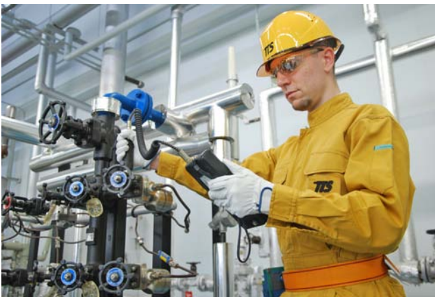
Figure 13.2. The steam trap survey is the key component of a steam trap management program. However, a plant should not jump into performing the survey without proper planning and preparation. (Courtesy TLV Corporation. All rights reserved.)
