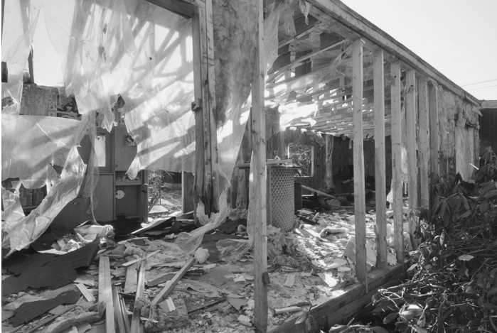
Figure 12.7 There was significant destruction or damage to the housing populations after Hurricanes Rita and Katrina. (Source: FEMA/Hans Pennink.)
