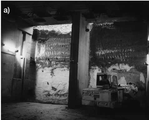
Figure 5.80 a) Excavating the lower half of a 10 m high face through frozen, waterbearing sands and gravels, and b) Webster Schaeff excavating machines used on the Boston jacked box tunnels (Clayton et al. 2001) (courtesy of BAM Nuttall Ltd and John Ropkins Ltd)
