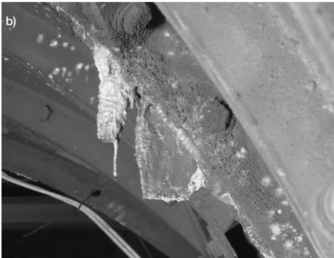
Figure 8.13 a) Existing Piccadilly Line tunnels, SGI-Segments (LHS), Concrete Segments (RHS), b) existing Piccadilly Line Eastbound Tunnel, stalactites on the SGI-Segments
