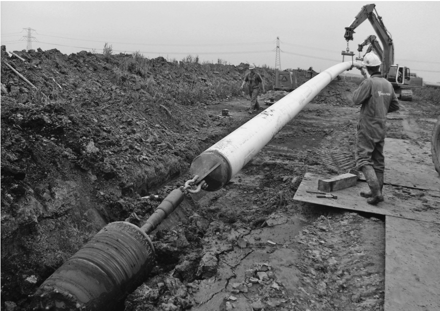
Figure 5.89 Pullback operations showing back reamer and final pipe (courtesy of Prime Drilling HDD-Technology)
