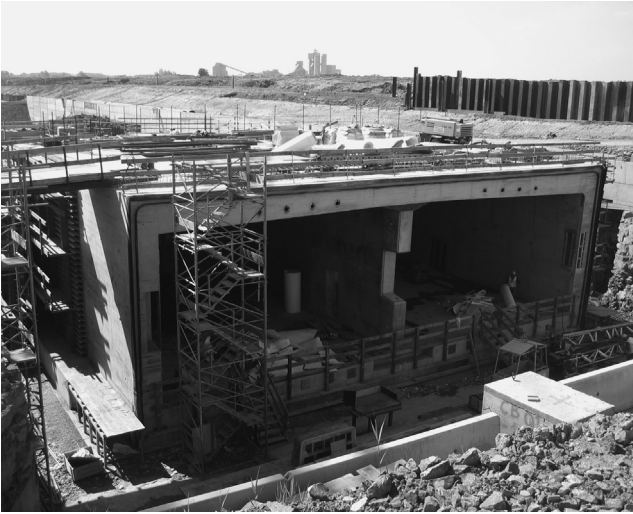
Figure 5.64 Construction of one of the elements for the Limerick immersed tube tunnel in Ireland (courtesy of COWI A/S)
