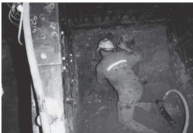
b) Hand mining in a top compartment through very weak, loose sand and silt
