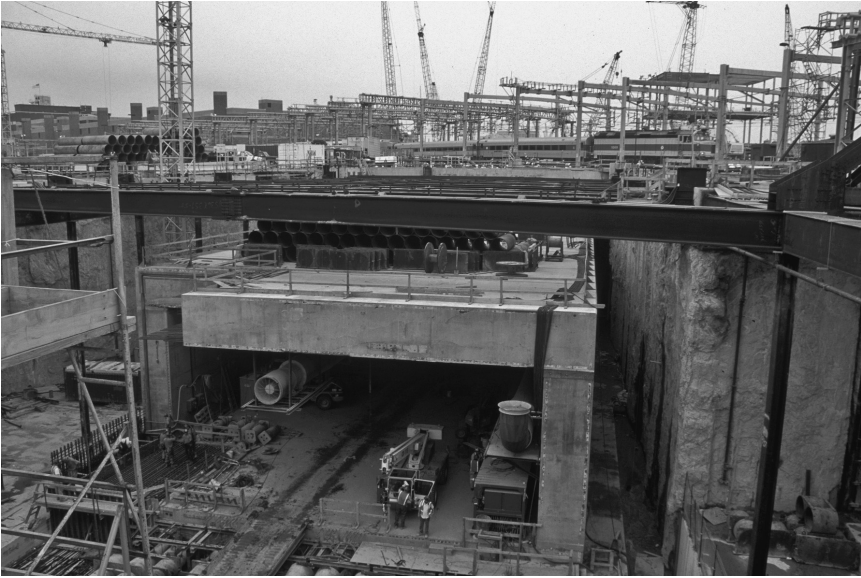
Figure 5.78 One of the jacked box tunnels during the jacking process, note the cover depth above the tunnel and rail road lines at the ground surface (courtesy of Massachusetts Turnpike Authority)
