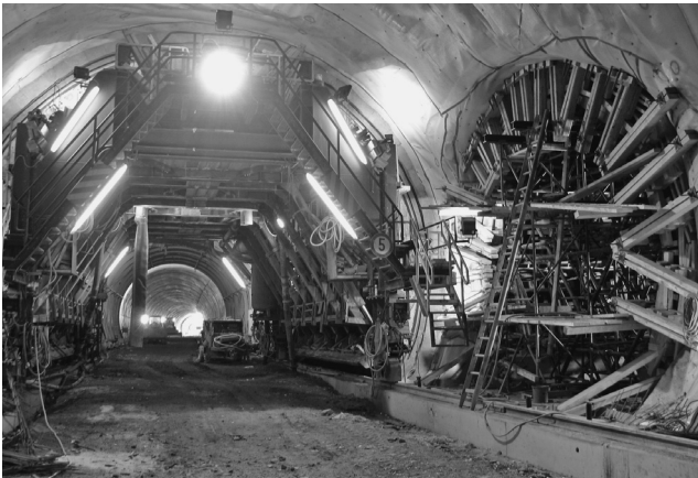
Figure 4.29 Inner lining construction, including waterproofing as used for the emergency cross-passage, Heidkopf Tunnel, Germany (courtesy of ALPINE BeMo Tunnelling GmbH Innsbruck)
