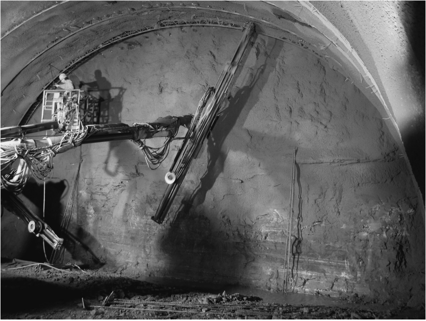
Figure 4.9 Anchor installation associated with sprayed concrete lining, HKT Tunnel, Germany (courtesy of ALPINE BeMo Tunnelling GmbH Innsbruck)
