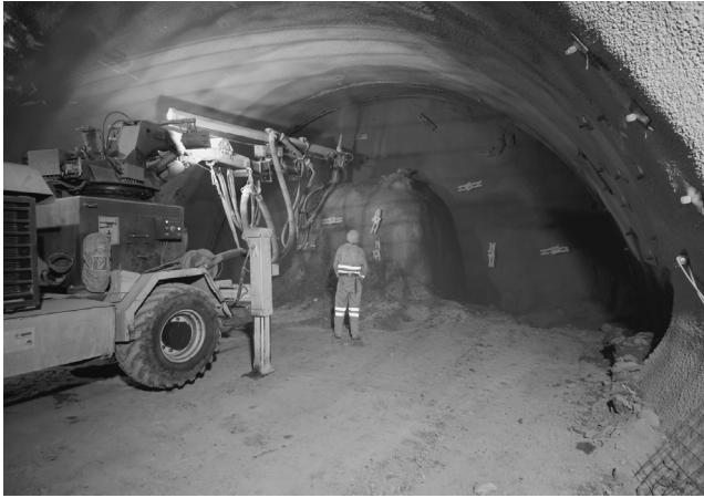
Figure 4.13 Installation of temporary dowels into the tunnel face during the construction of the Lainzer Tunnel LT31 in Vienna, Austria
