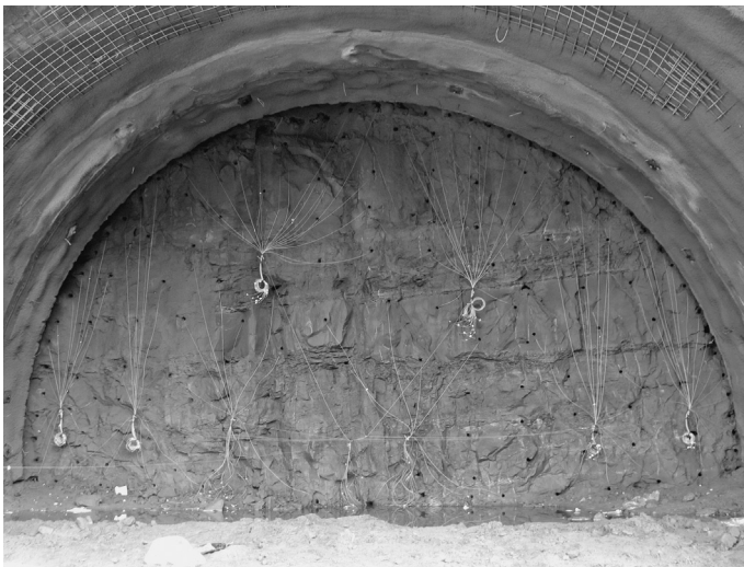
Figure 5.41 Example of a face ready to blast in the Heidkopf Tunnel, Germany
