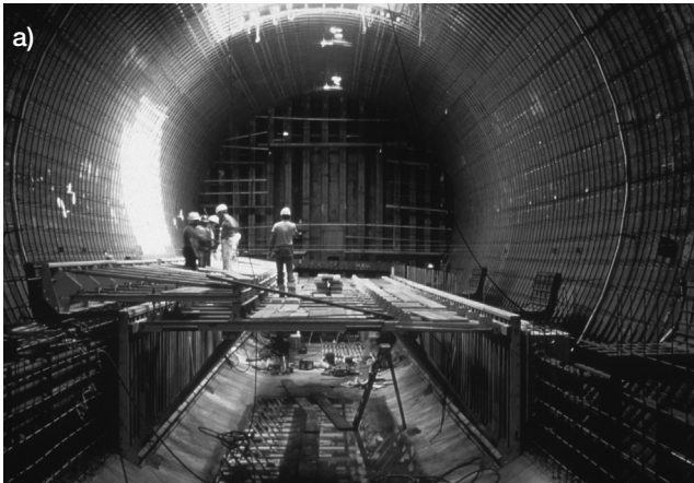
Figure 5.68 a) Internal fitting out of one of the tunnel elements (a reinforced concrete lining was placed inside the steel shell), b) the binocular immersed tube emerging into the cut-and-cover section of the Ted Williams Tunnel (courtesy of Massachusetts Turnpike Authority)
