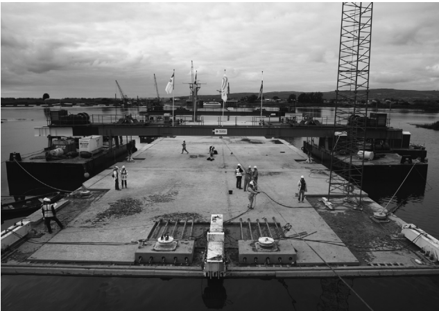
Figure 5.65 One of the elements for the Limerick immersed tube tunnel being towed into position ready for sinking (courtesy of COWI A/S)
