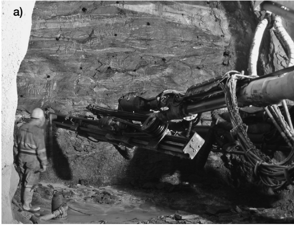
Figure 5.36 Examples of drilling blasting holes, a) and b) for an emergency cross passage, Katschberg Tunnel, Austria, c) for the Spillvatten Tunnel, Goeteborg, Sweden (an 8 km sewer tunnel, cross sectional area 11 m 2 , ground included granitic gneiss)
