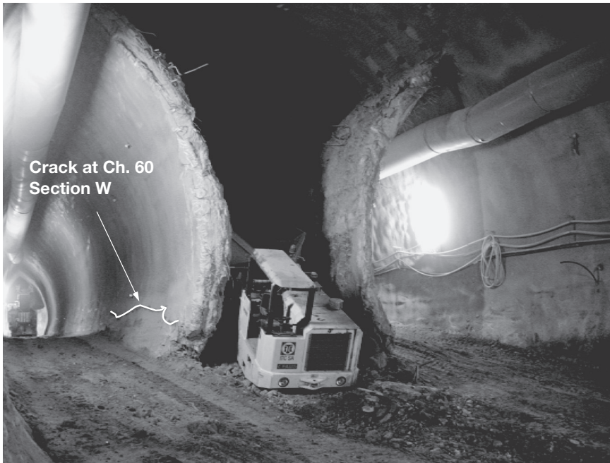
Figure 8.24 Crack in the inner wall of the side wall drift, section W, Chainage 52–60
