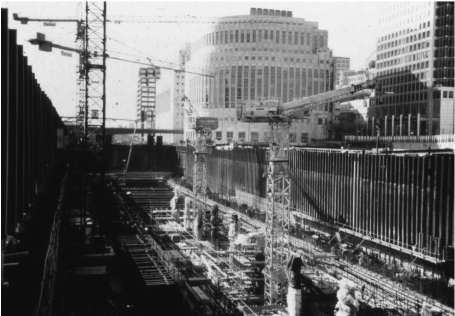
Figure 5.51 Canary Wharf Station during construction on the London Underground Jubilee Line Extension, UK
