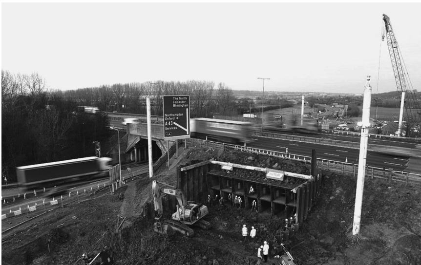
Figure 5.76 Completion of the jacking process showing the shield (Allenby and Ropkins 2004, courtesy of BAM Nuttall Ltd and John Ropkins Ltd)
