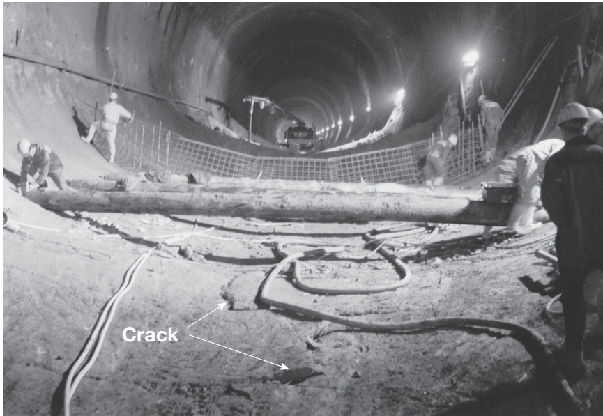
Figure 8.2 Contingency measures in the form of tree trunks at the completed cross section due to cracking after removing the backfill
