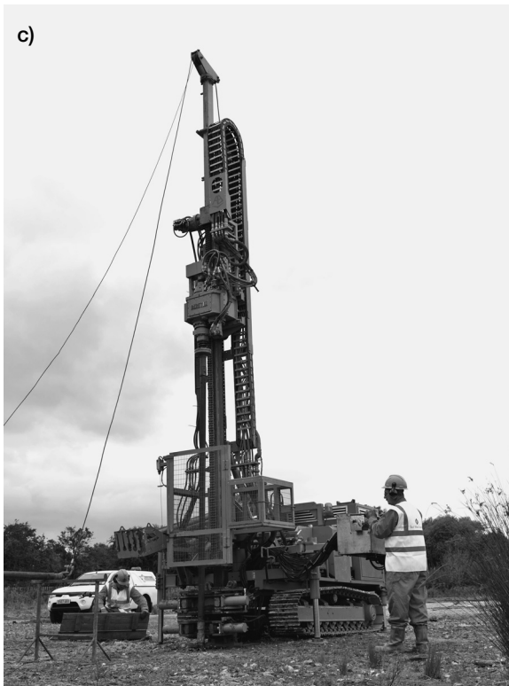
Figure 2.4 a) and b) Cable percussion rig and c) rotary drilling rig (courtesy of Soil Mechanics)
