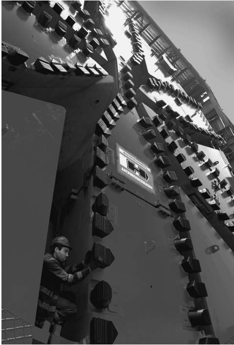
Figure 5.23 Cutter dressing used on a Mixshield TBM in Shanghai through sand, clay and loose gravel/boulders (courtesy of Herrenknecht)
