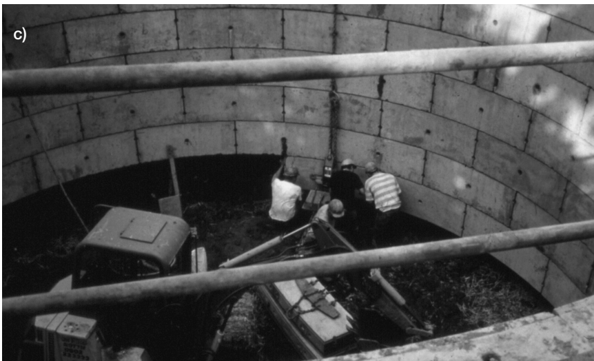
Figure 4.26 (continued) An example of the ‘underpinning’ technique used to construct a shaft, b) shows the excavation process, and c) shows the installation of the concrete segments
