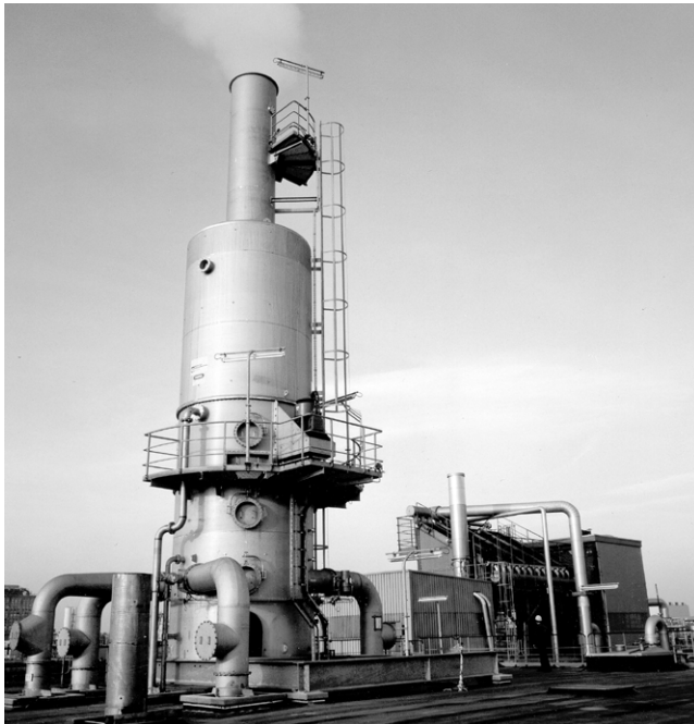
Figure 11.4 Rotary scrubber (Trema Verfahrenstechnik GmbH).
