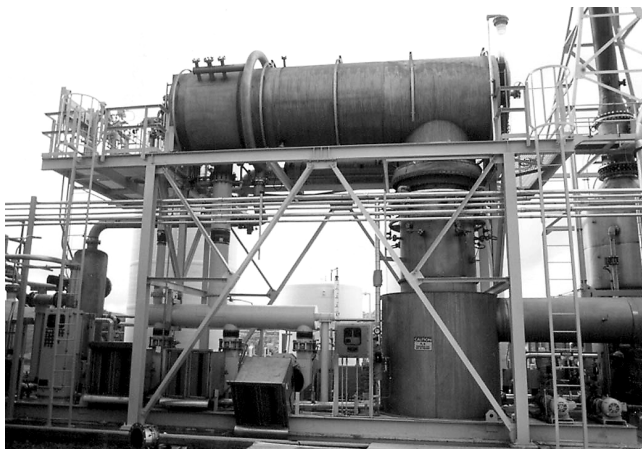
Figure 16.2 Thermal oxidizer for VOC control (Banks Engineering, Inc.).
