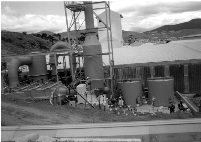
Figure 14.4 Preformed spray scrubber on superphosphate dryer (Bionomic Industries Inc.).
