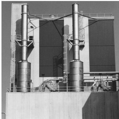
Figure 18.4 Vane type scrubber installation (Entoleter, Inc.).
