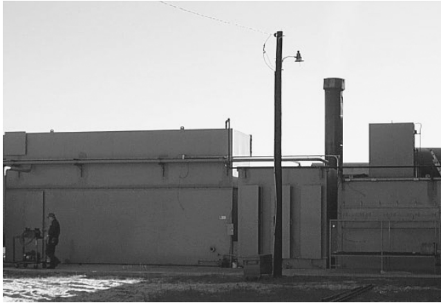
Figure 8.4 With prefilters, water cooling coils on curing ovens (Advanced Environmental Systems, Inc.).
