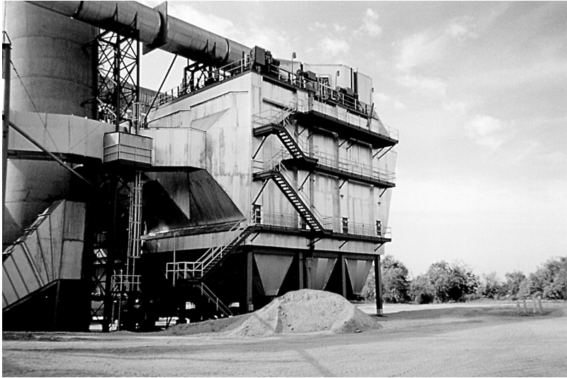
Figure 5.1 Typical electrostatic precipitator in operation (BHA Group, Inc.).
