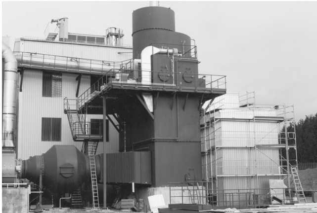
Figure 20.3 Particle board dryer WESP (Geoenergy International, Corp.).
