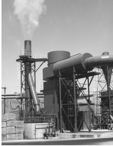
Figure 20.2 WESP on veneer dryer (Geoenergy International, Corp.).
