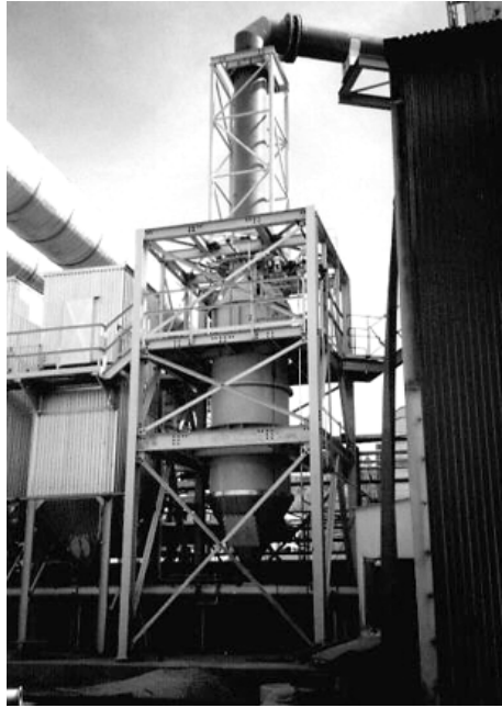
Figure 6.8 Evaporative cooler on aluminum plant (Hart Environmental, Inc.).
