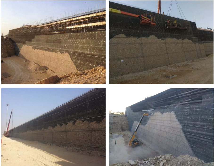
Fig. 13. Filling of stone between wrap around GRS and steel mesh to form Muralex facing
