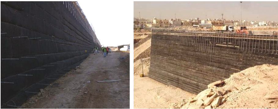
Fig. 11. Wrap around wall, during construction prior to installation of Muralex facing; anchoring bars visible
