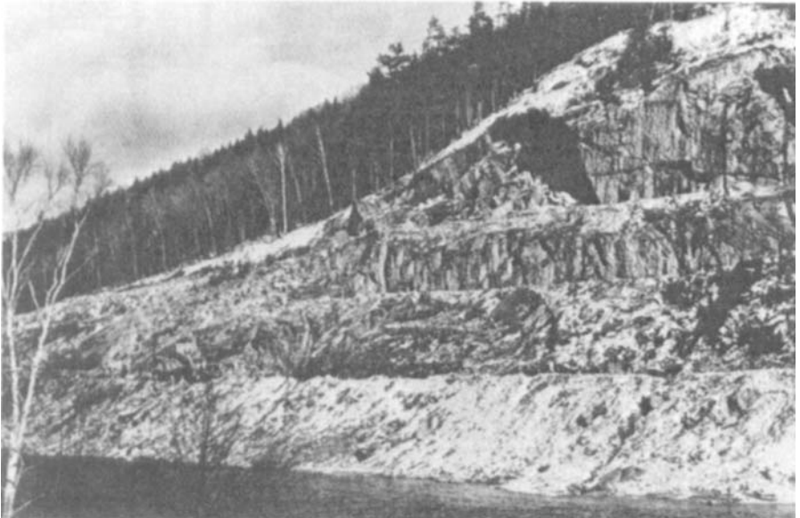
Figure 9-53 Slope failure during construction of I-93 in Woodstock, New Hampshire. (From Fowler, 1976. Reproduced by permission of ASCE.)
