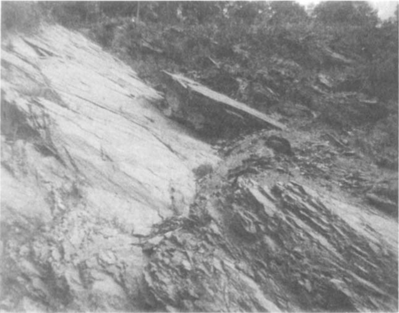
Figure 9-19 Rock block sliding on planar surface.
