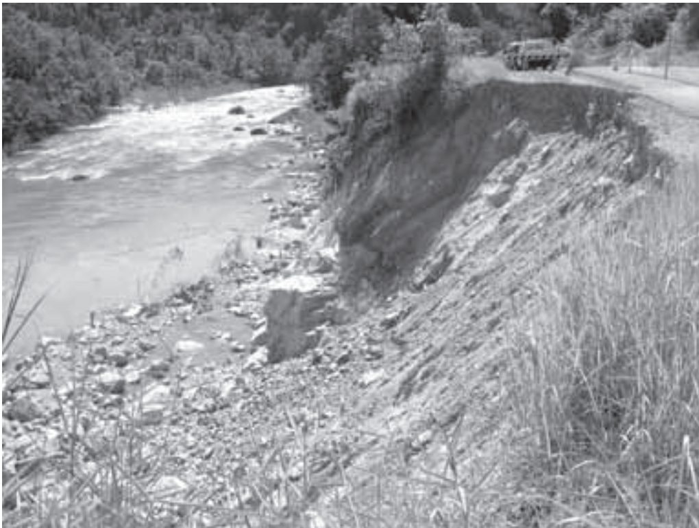
Figure 15.1 A slope failure (Courtesy of Dr. Kirralee Rankine, Golder Associates, Australia)
