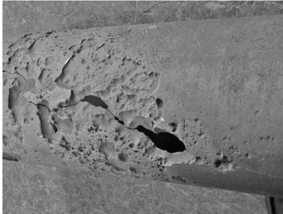
PHOTO 7.8 Selective leaching of a buried pipe.
