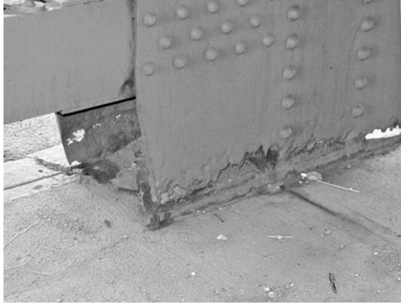
PHOTO 7.2 Moisture and contaminants present in the debris around this bridge support lead to the attack.
