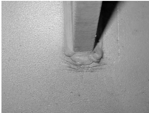
PHOTO 4.7 The cracked paint shows proof of the deformation that took place when this crane beam was overloaded.
