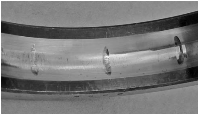
PHOTO 10.27 This false brinelling resulted from long-term vibration while the bearing was not rotating.
