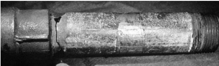
PHOTO 7.5 Galvanic corrosion of a steel nipple connected to a bronze valve.
