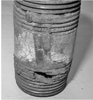
PHOTO 7.6 This steel nipple was originally in the case iron pump housing shown in Photo 7.7. It corroded as the anode in a galvanic circuit.
