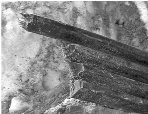
PHOTO 9.2 The instantaneous failure of a group of four belts. The fact that there is absolutely no fraying of the tension members tells us that the failure happened very rapidly. This is similar to an overload failure of a metal piece and tells us that the physical cause of the failure was present immediately before the failure occurred.
