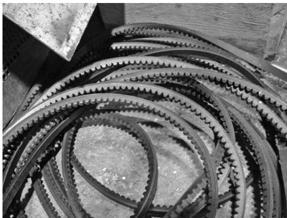
PHOTO 9.5 This is a pile of belts that has just been removed from a large fan. The elastomer on the sheave contact surfaces is shiny and polished, proof that the belts have been slipping.
