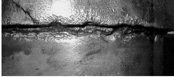
PHOTO 7.15 Pitting corrosion adjacent to the weld on a steel elevator cylinder — caused by the residual stress.
