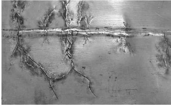
PHOTO 7.20 SCC on the outside of a milk storage tank.
