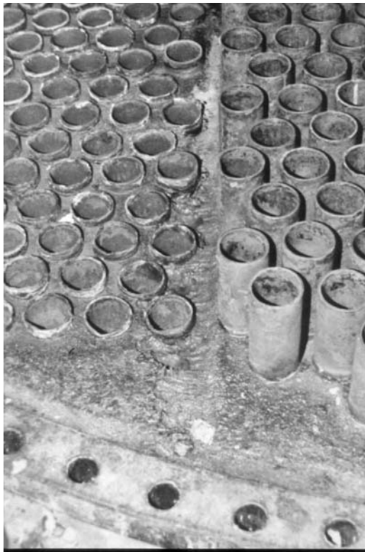
PHOTO 7.3 The increased velocity under the baffle plate on this heat exchanger caused increased corrosion rates.
