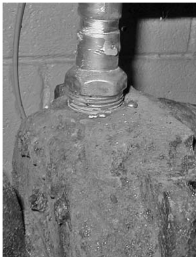
PHOTO 7.7 By making the large cast iron part the anode, the assembly life is increased tremendously.
