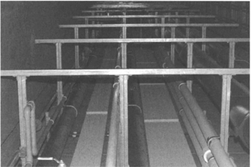
FIGURE 25.5 Process piping supports.
