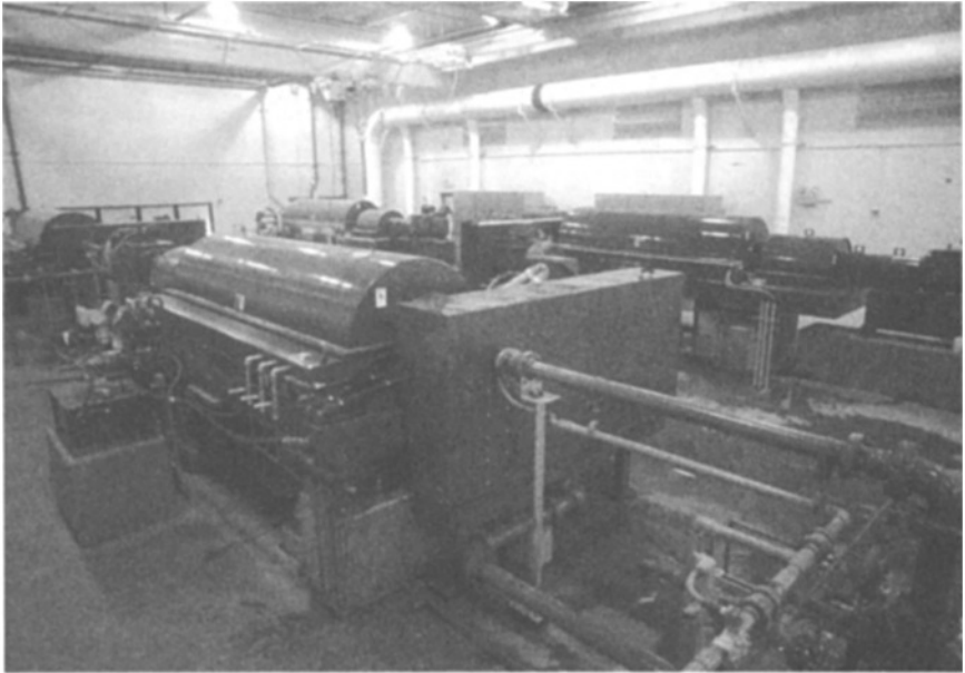
FIGURE 17.24 Centrifuge system. (Courtesy of City of Phoenix Water Services Department.)
