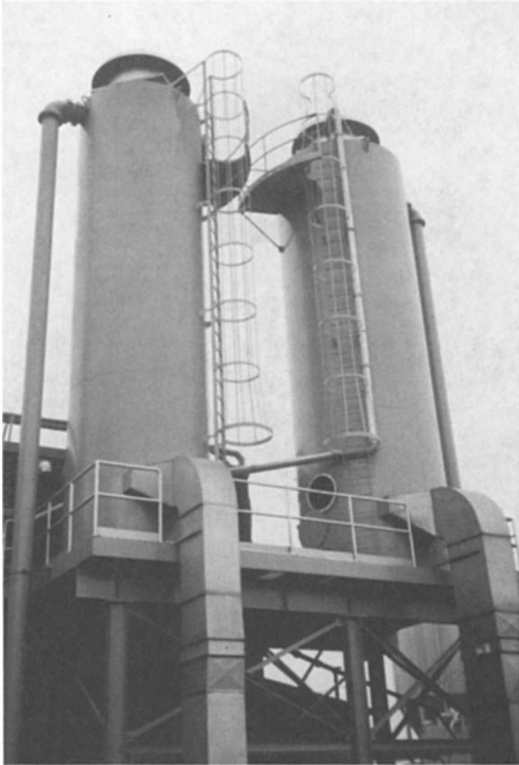
FIGURE 5.2 View of a packed column installation. (Source: U.S. Environmental Protection Agency.)
