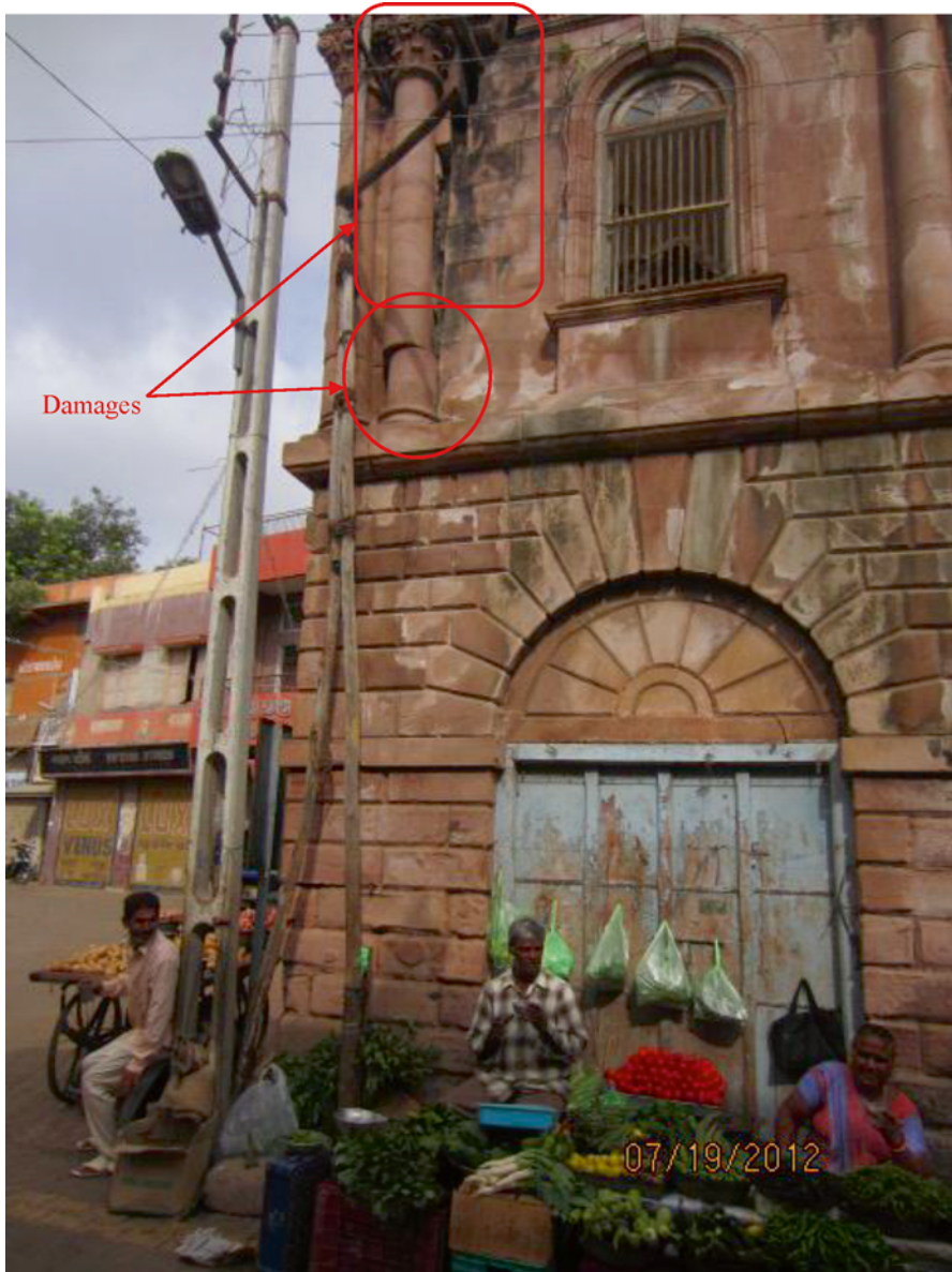
Fig. 6.11 Vegetable sellers in Bhuj sitting next to a damaged building (Source: Author 2012)
