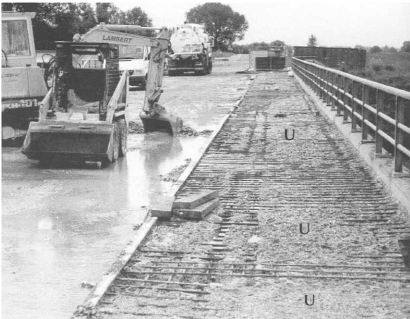
Figure 2.21 Threshold situation in a hydrodemolished concrete substrate (photograph: Aquajet Systems AB, Holsbybrunn)
