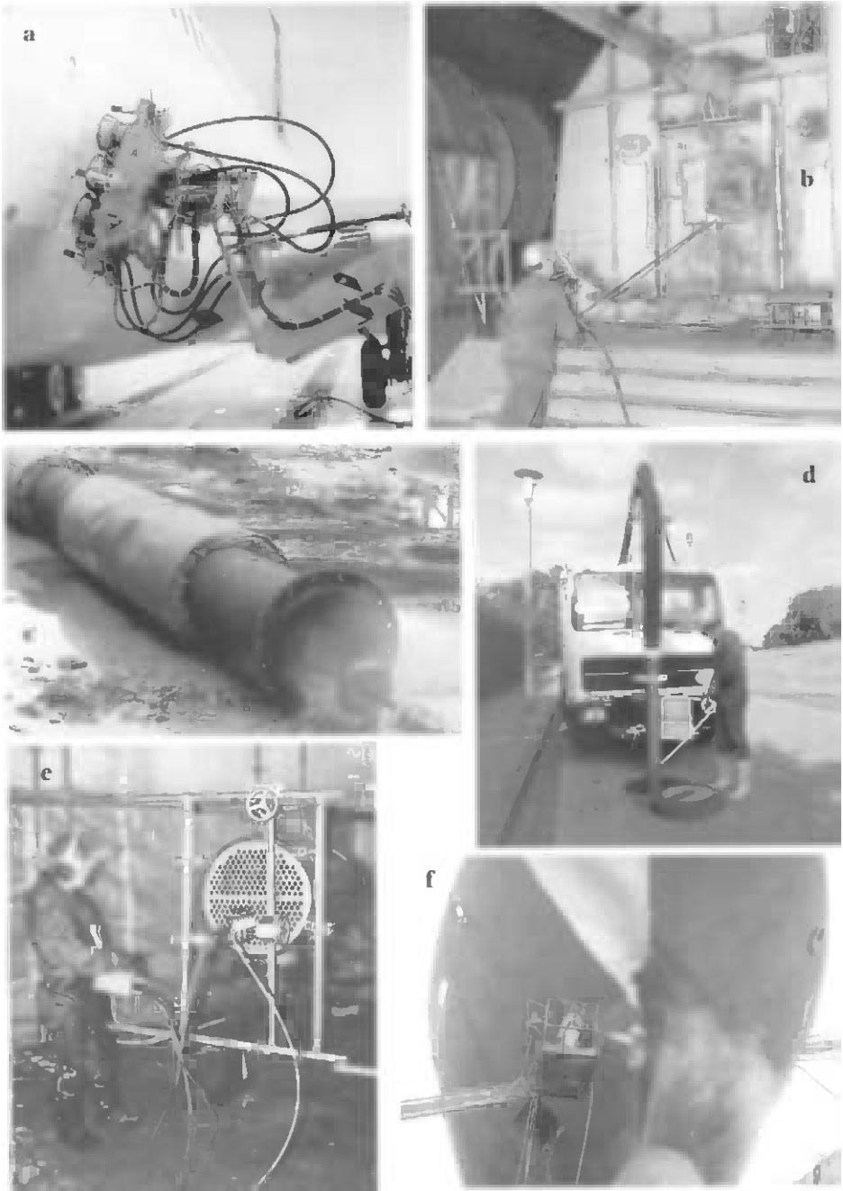
Figure 1.6 Industrial cleaning applications of water jets (a) aircraft cleaning (WOMA GmbH, Duisburg); (b) cement kiln cleaning (WOMA GmbH, Duisburg); (c) pipe cleaning (WOMA GmbH, Duisburg); (d) sewer cleaning (WOMA GmbH, Duisburg); (e) tube bundle cleaning (WOMA GmbH, Duisburg); (f) coating removal with UHPAB for steel surface protection (Mühlhan Equipment Services GmbH, Hamburg)
