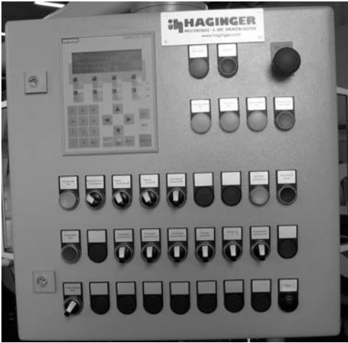
Fig. 6 Panel of a PLC based control system
