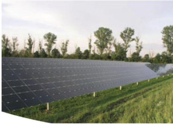
Fig. 4.2 Large PV power plant with thin film solar modules
