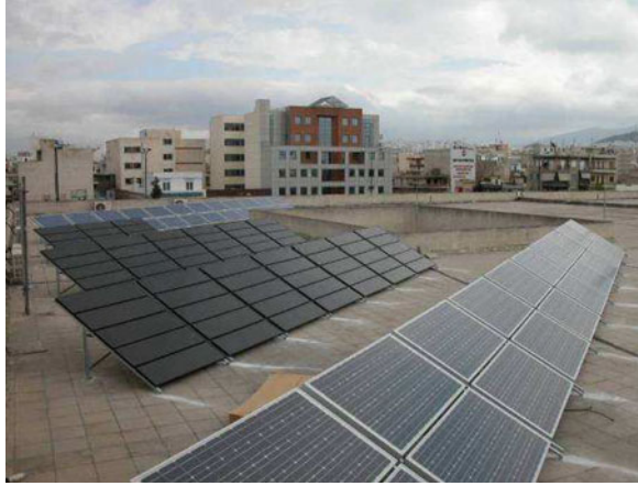
Fig. 5.8 PV roof mounted and grid connected
