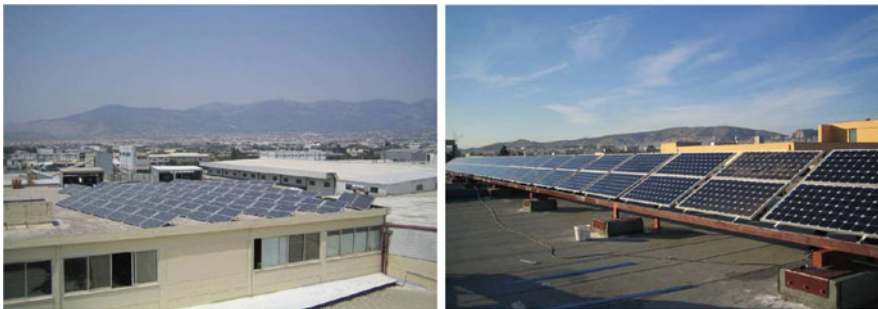
Fig. 6.1 PV panels' roof mounted at industrial building (Milk Dairy Industry)
