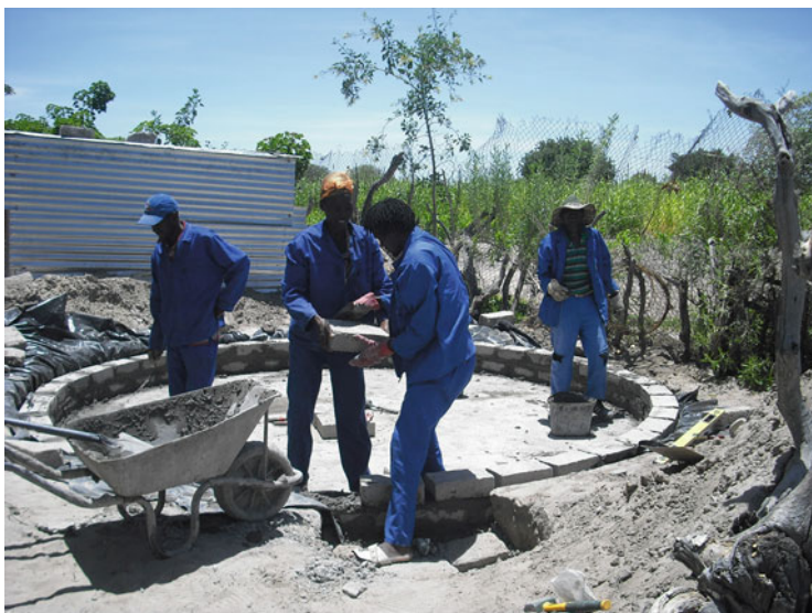
Fig. 16.2 Trained technicians during the construction of the concrete brick tank for rainwater in the village of Epyeshona
