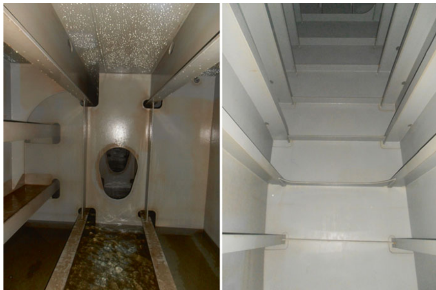
Fig. 2 Interior of a DBT ( left ) and ST ( right ) ballast tank on a bulk carrier (Photos: Guy Mali)
