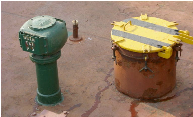
Fig. 6 An air-vent on the left , a sounding pipe in the center back , and a TST hatch on the right on a bulk carrier
