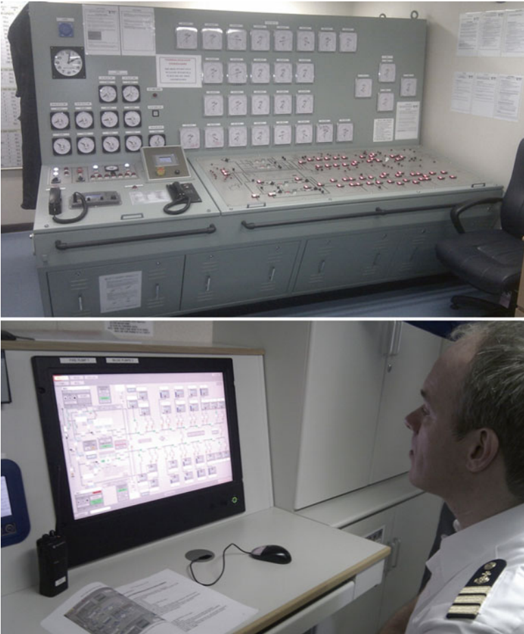
Fig. 8 Ballast control console ( top ) and computer ballast system control ( bottom )
