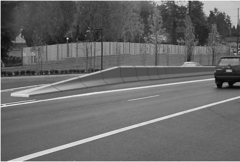
Figure 13.14 Low-speed terminal for rigid barriers. (From Bligh R et al., Median barrier guidelines for Texas . Texas Department of Transportation, Austin, 2006.)
