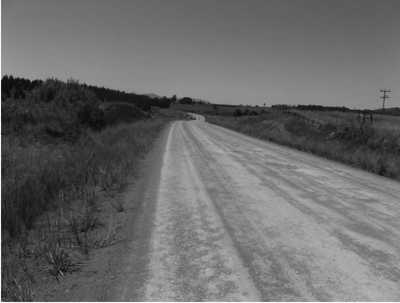
Figure 12.1 Typical unpaved road. (Photo: RC Burrell.)
