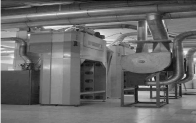
FIGURE 1.16 Contamination clearer attached in blow room line.
