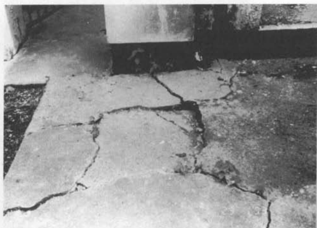
Figure 8-3. Pavement cracking over expansive soil.
