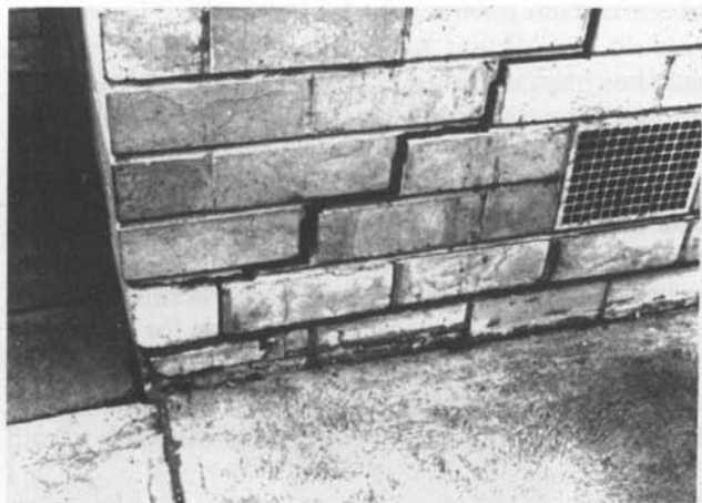
Figure 8-2. Expansive soil and building wall.
