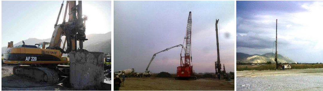
FIG. 7a, 7b and 7c Construction of the bored piles (left-center) and jet grout columns (right)
