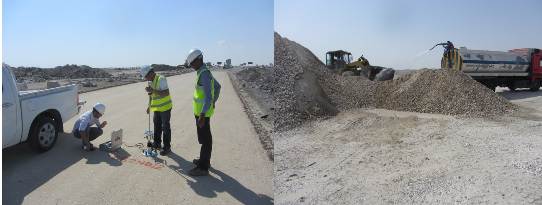
FIG. 4. (a) Lightweight deflectometer testing on EW+DS; (b) Adding water to CC prior to compaction
