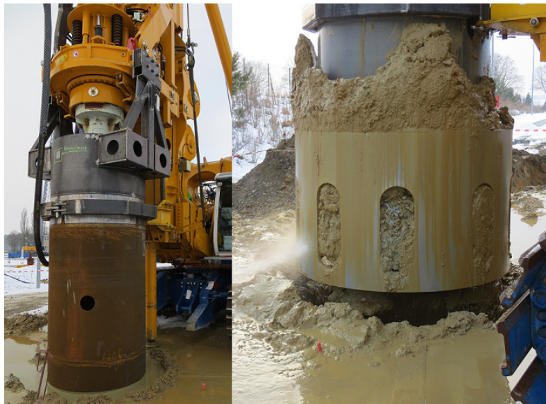
FIG. 2. The MIDOS pile during the in situ tests in South Germany (left) and the mixing chamber after the installation (right).
