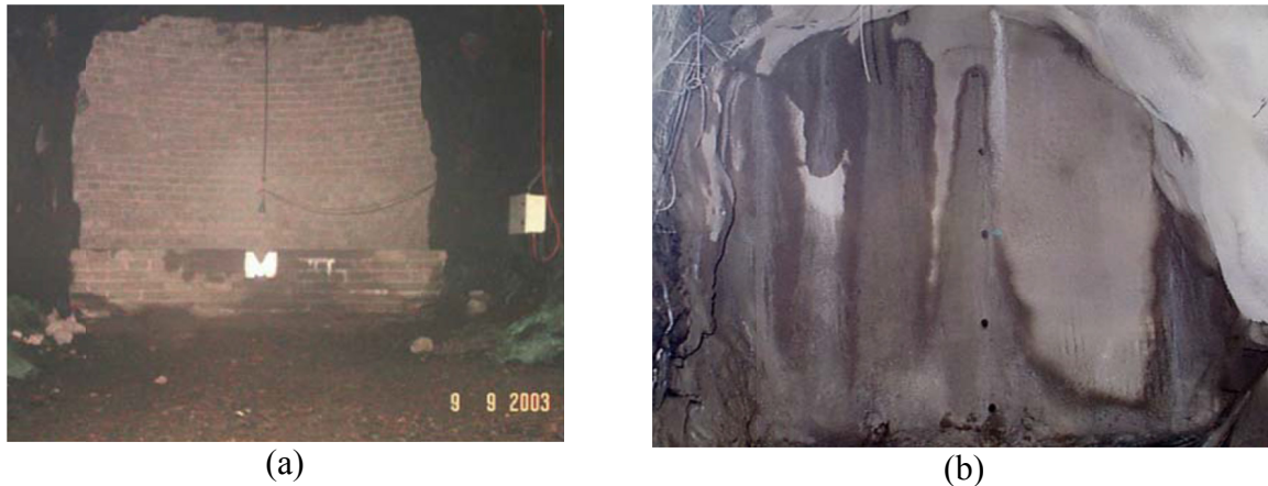
FIG. 1. Examples of barricade: (a) permeable brick barricade in place (adopted from Berndt et al. 2007) and (b) typical sprayed shotcrete/fibrecrete paste barricade (adopted from Revell and Sainsbury, 2007)
