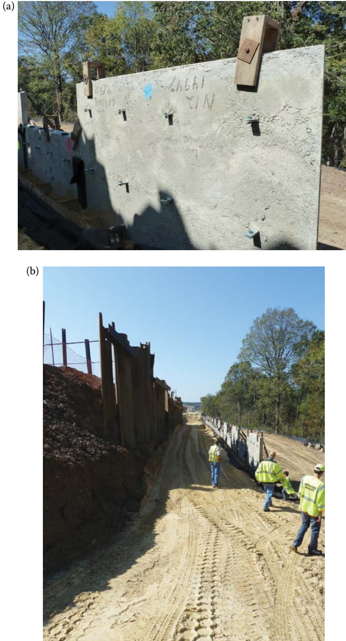
FIGURE 6.12 (a) MSE wall construction concrete panel with ties for the metal strips. (Credit: A. Braham.) (b) MSE wall construction overview with select fill. (Credit: A. Braham.)
