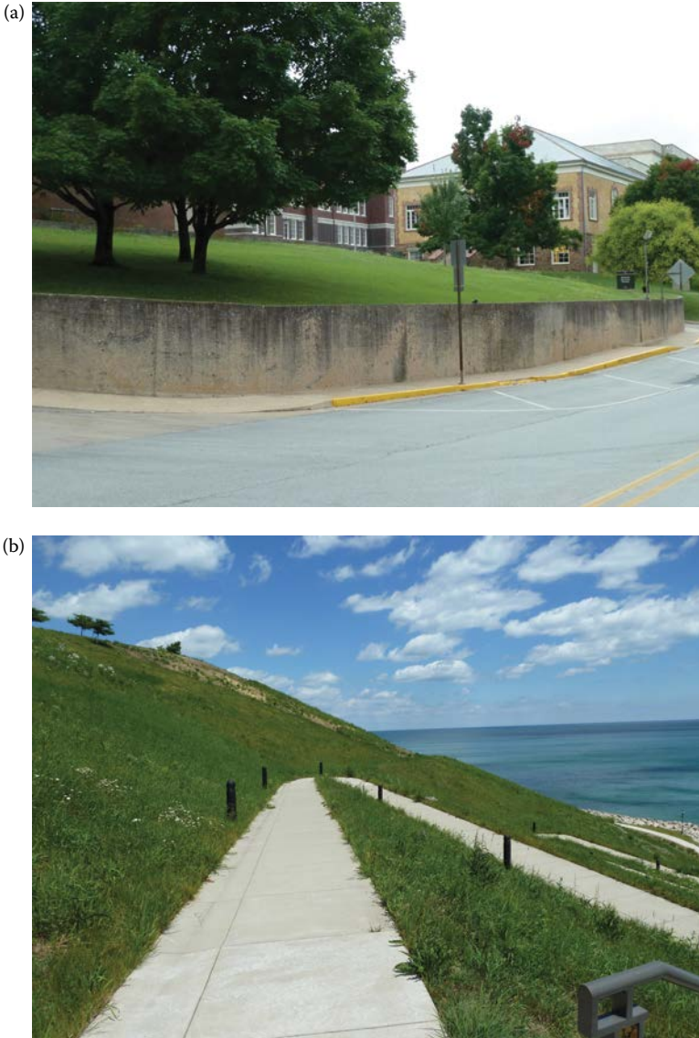
FIGURE 6.4 (a) A traditional concrete retaining wall on the University of Arkansas campus. (Credit: A. Braham.) (b) A bioengineered slope just north of Milwaukee, Wisconsin. (Credit: A. Braham.)
