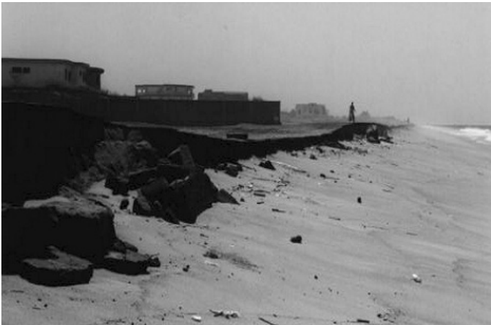
Figure 5.6 An undermined (lateritic) beaten earth road in Cotonou showing an erosion micro-cliff (about 1m high) at the top of the beach, generated by the rapidly retreating shoreline
