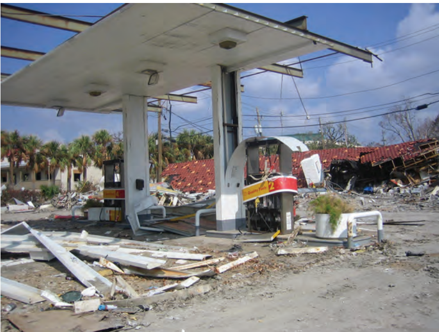
Figure 11.8 Filling station (post-Hurricane Katrina).
