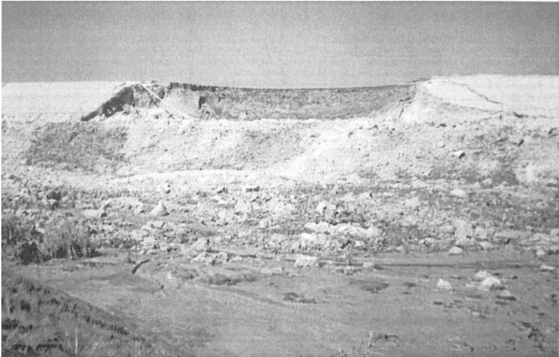
Figure 10: (b) View of failure of Simmergo tailings dyke.
