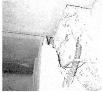
Figure 6: Damaged Column due to Lateral Heave.
