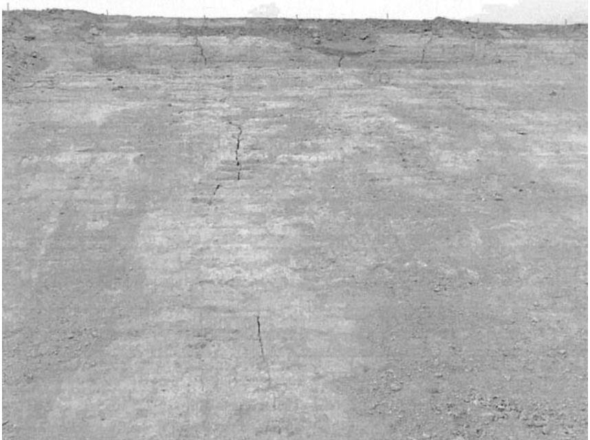
Figure 7. Upstream slope of flood retention structure in arid environment in central Arizona with upper 1 m (3 ft) of material removed. Note visible transverse cracking extending from crest. This FRS had a central drain installed with deep trenching at the crest in conjunction with embankment crack mapping in the early 1980's.
