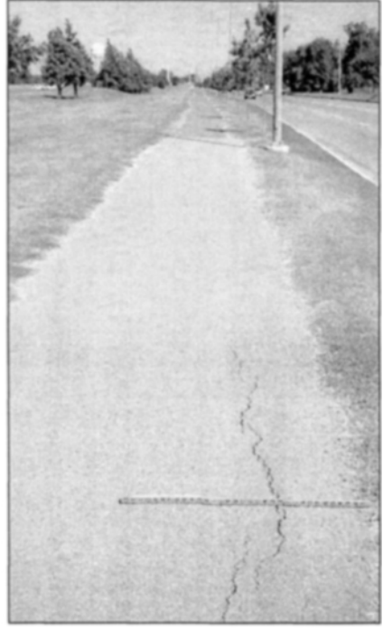
Figure 2b. Control section with longitudinal cracks, looking east.
