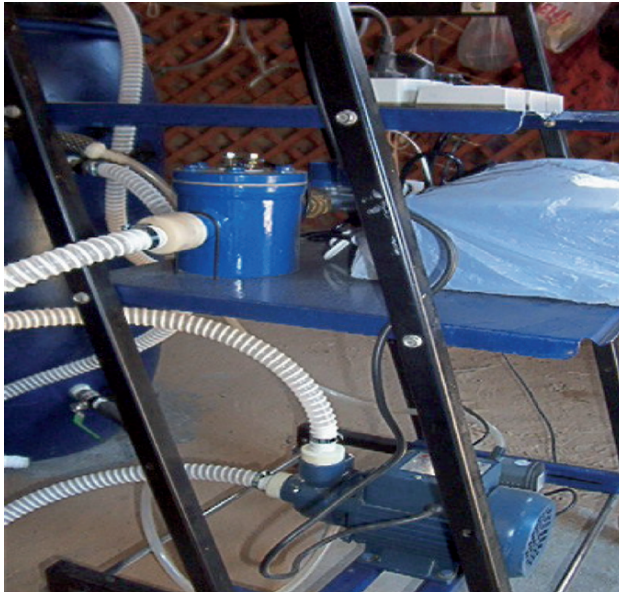
Figure 3. The disinfection device installed in water desalination systems with solar cells
