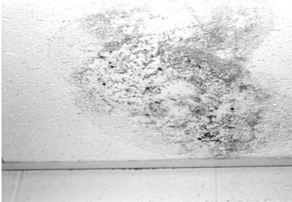
Figure 6.9 Stachybotrys and other mold species growing on ceiling tile.
