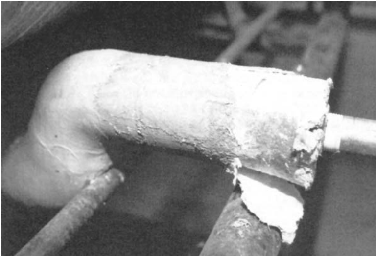
Figure 2.3 Partially damaged thermal system insulation containing asbestos.
