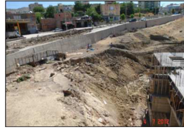
Figure 2. Sliding land soil and foam concrete landfill study area.
