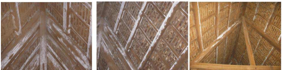
Figure 6. Detail of the fungi infestation found in the west wing of the museum roof.
