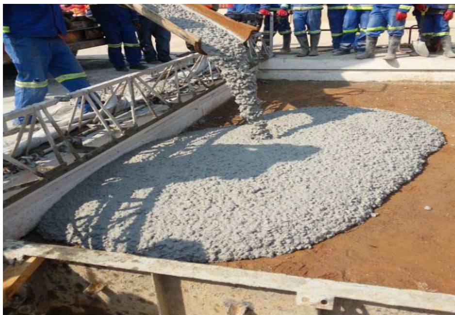
Photo 1. Application of Geopolymer concrete on site at Transnet’s City Deep Container Terminal.
