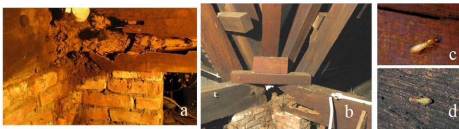
Figure 3. a) head of a beam decayed by termites; b) head of a beam completely destroyed by termites, c),d) Coptotermes Gestroi individuals.
