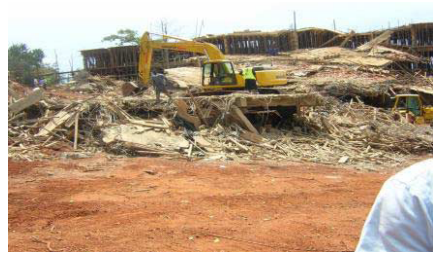
Figure 2. BBJ building collapse, Uganda [1]
