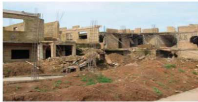
Figure 1. Collapsed part of the building
