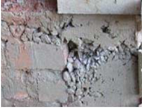
Figure 3. Honey-combed concrete at the column base [11]
