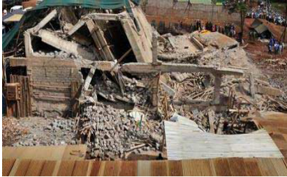
Figure 1. Building collapse in Kiambu District, Kenya
