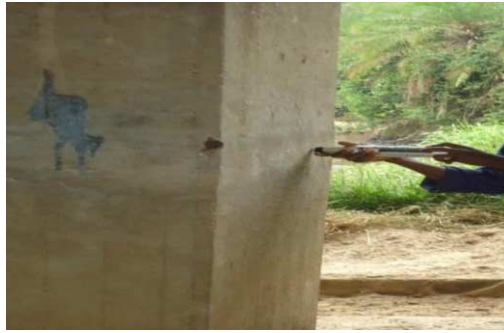
Figure 2. Schmidt Hammer test is done horizontally on a pier column, just above the flood level
