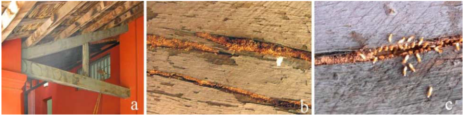
Figure 5. Colonnade beam: a) fungi signs; b) termites pathways; c) living termites.
