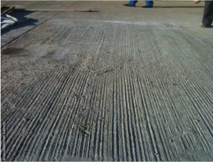
Photo 2. Geopolymer concrete on site at the City Deep Container Terminal after 3 days
