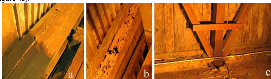
Figure 4. a) termites pathways on a roof bearing beam; b) the same beam after the removal of wood surface; c), horizontal prop beam collapsed due to termites infestation.
