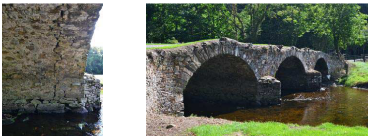
Figure 4. Longitudinal cracking in Woodhouse Bridge
