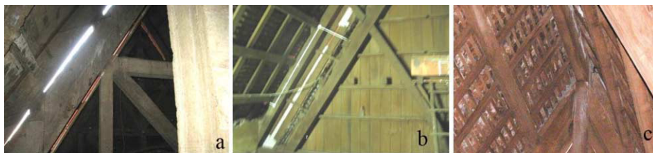
Figure 7. Roof structure: a) open gap between the folds of the roof; b) open gap between the folds sealed with tape; c) open gap between the folds sealed with mortar.
