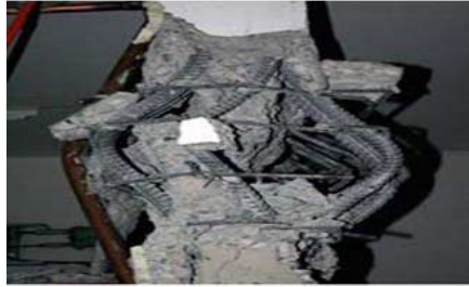
Figure 5. Buckling failure of the under-designed column [1]
