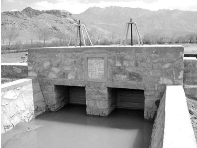
FIGURE 22.6 A typical gate fitted canal intake.
