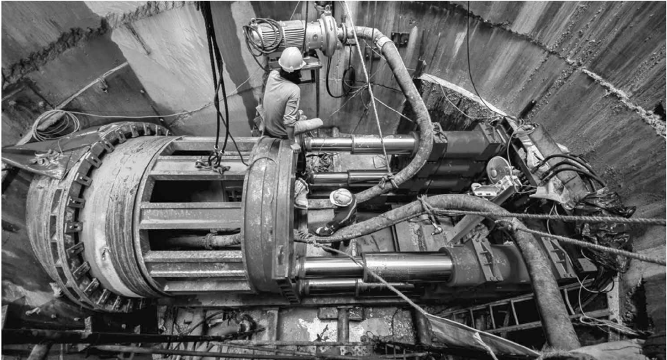
FIGURE 26.5 Slurry microtunneling at 14 m depth (water transmission pipelines from east side of Chao Praya river to the Bang-Pra reservoir). (Courtesy of Thai Triumph, 2015.)
