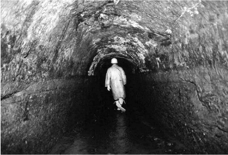
FIGURE 21.7 Inside of the Tatsumi Tunnel (favorable ground) (From HP/Wikipedia, Tatsumi Aqueduct, 2015a. With Permission.)
