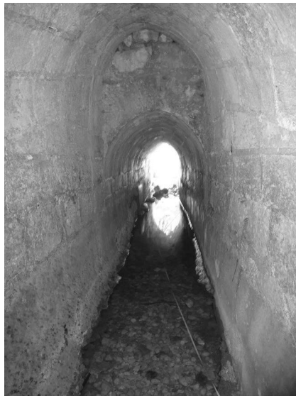
FIGURE 10.11 Tanur spring. A built spring tunnel from perfectly carved ashlar. (Photography by Yechezkel.)
