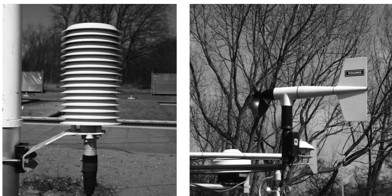
Figure 5.3 Details of a rain gauge and wind sensor.
