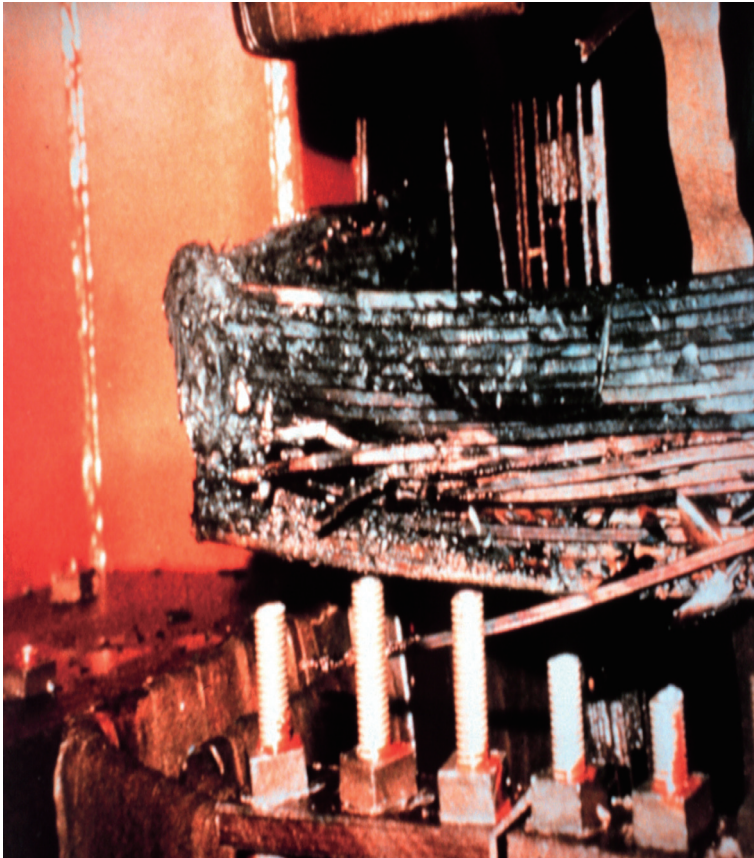
Plate 10 A closeup picture of one of the transformers melted by the electrical overload brought about by the great geomagnetic storm of March 1989 (from the National Space Weather Program Strategic Plan, Office of the Federal Coordinator for Meteorological Services and Supporting Research, FCM-P30-1995, Washington, DC, 1995).
