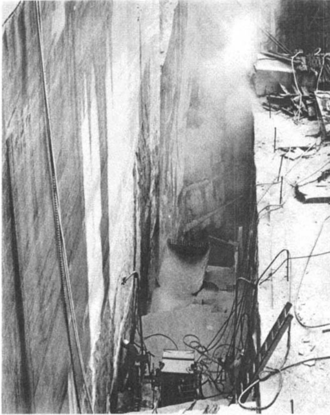
Figure 25.6 Channel burning in a granite quarry. The burner, suspended from a boom, is cutting deep in the kerf. The dust and burner emission plume is visible in the upper right hand corner.
