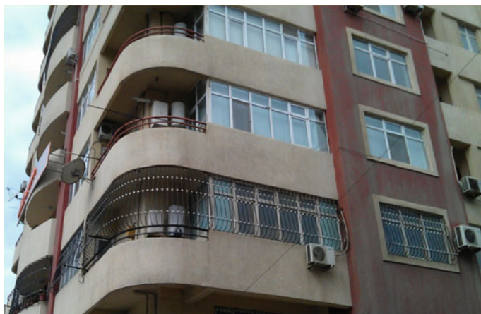
Fig. 17.1 Small boilers on the balcony of an apartment building to heat individual apartments
