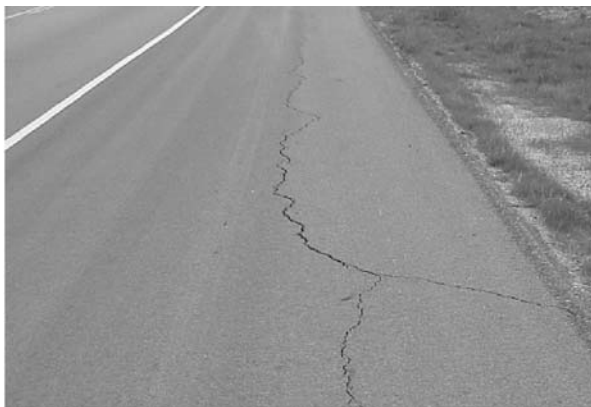
Figure 18.1 Photograph showing propagation of cracks from sub-grades to the adjacent pavement.
