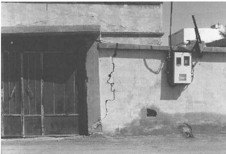
Figure 19.3 Cracks in a reinforced concrete gate and adjacent wall.
