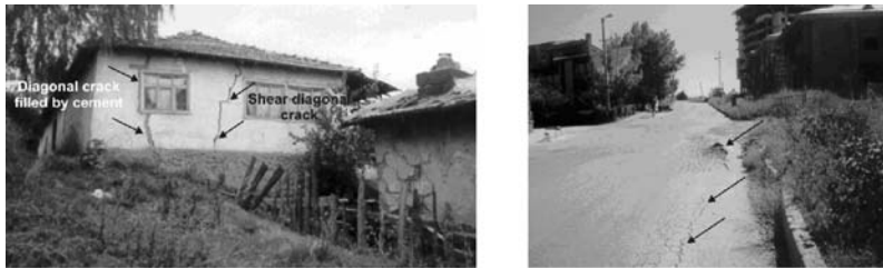
Figure 22.1 (a) A typical damaged one-storey building, and (b) cracks and heave on the asphalt pavement due to expansion of the investigated soil.
