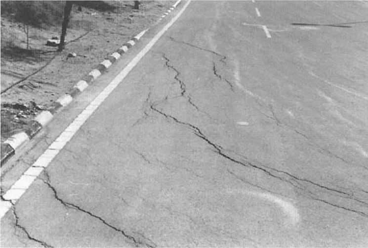
Figure 19.5 Cracks in a road pavement in the town.
