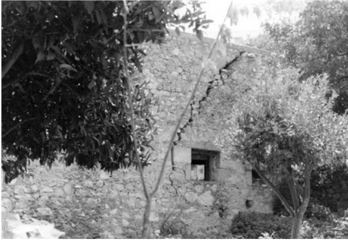
Figure 25.8 Example of structure damage caused by expansive soil (slab failure).
