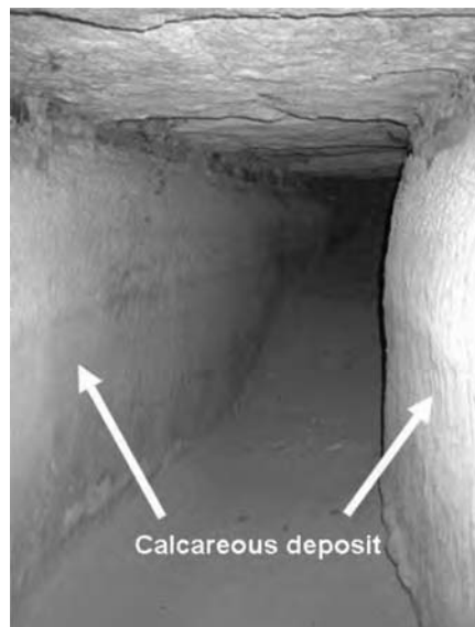
Figure 13.17 Picture taken from the inside of a masonry channel inside the city of Apamea. Calcareous deposits on the channel inner walls can be observed
