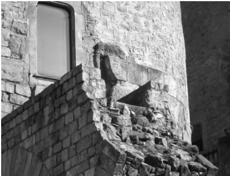
Figure 19.2 Rebuilt remnants of the Roman Aqueduct to Barcelona (with permission of M. Salgot)
