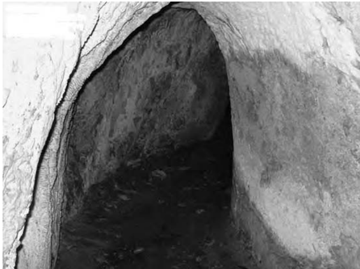
Figure 14.12 Remains of the tunnel of Roman aqueduct in Nikopolis (with permission of H. Gouvas)
