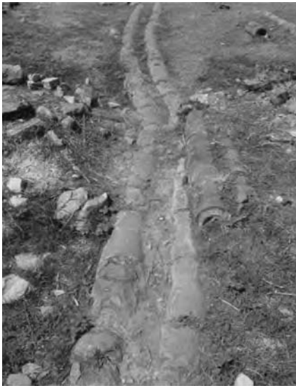
Figure 13.25 Pipelines starting from the water tower at the end of the Marnas aqueduct in Ephesus
