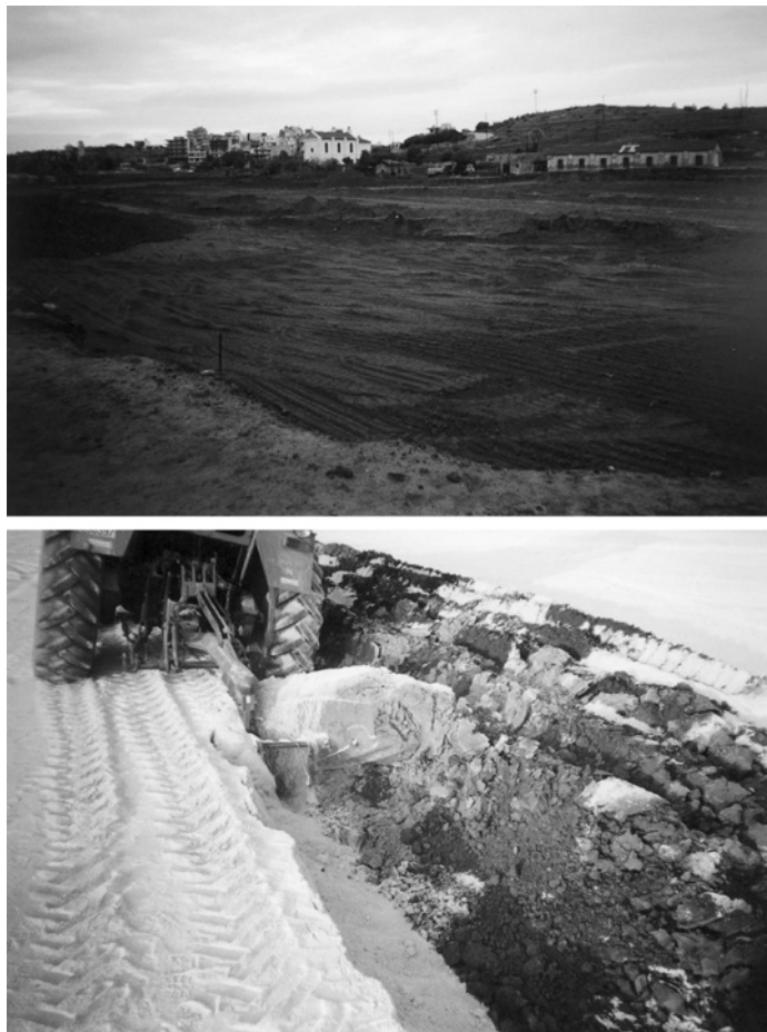
Figure 25.9 View of the ongoing works for the rehabilitation of the tailings dam in Lavrion (up) and amendment of tailings with ground limestone (down).
