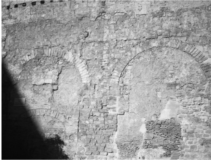
Figure 19.1 Badly preserved arches of the Roman aqueduct, Barcelona (M. Salgot, with permission).
