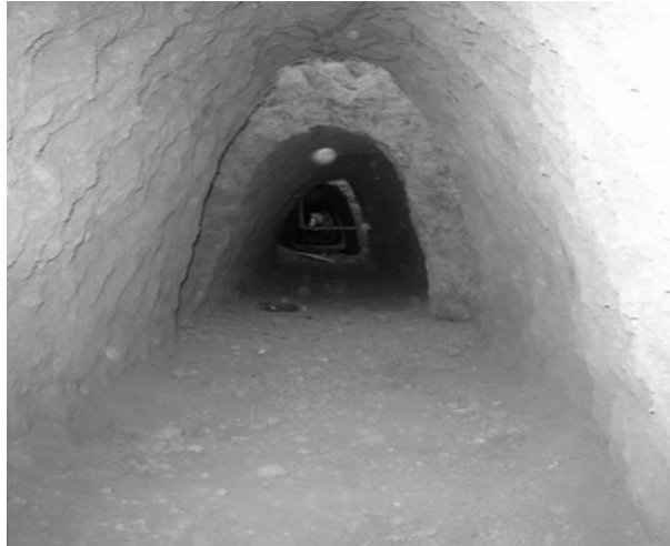
Figure 7.15 Execution of sewer lines by manually cut gallery. Neishaboor wastewater plan (with permission of NWWEC).
