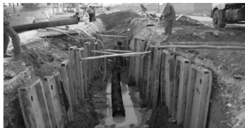
Figure 7.14 Open trench execution of wastewater line using wooden shields and sheet piles. Bushehr wastewater plan (with permission of NWWEC).
