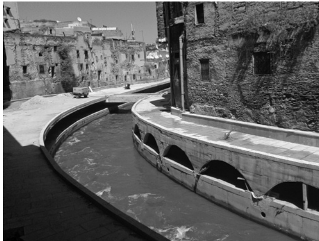
Figure 11.26 Two wastewater canals are being built along the river ‘Oued Fez’ (with permission of H. Benqilou).
