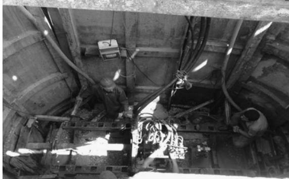
Figure 7.18 Execution of wastewater network by micro tunneling. Deilam wastewater plan (with permission of NWWEC).
