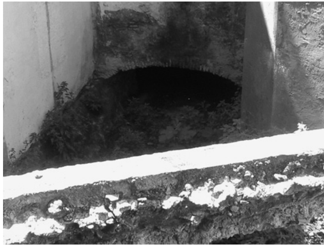
Figure 11.18 Traditional sewer under houses (with permission of H. Benqlilou).
