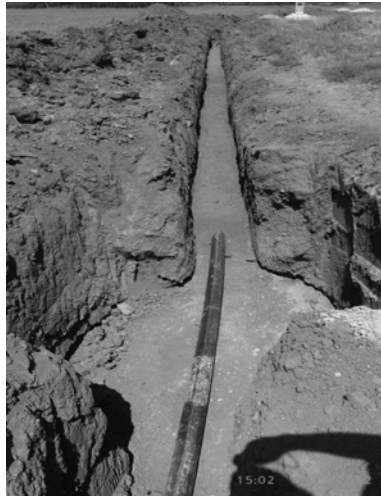
Figure 7.13 Open trench execution of wastewater line: The wastewater plan in the village of Abar from Sharood County (with permission of NWWEC).
