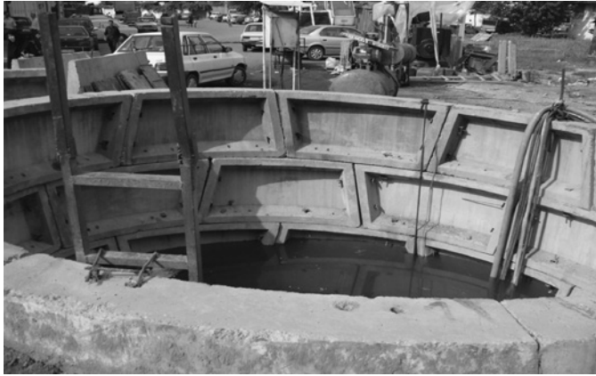
Figure 7.16 The application of prefabricated concrete segments in the send and receive shafts for pipe jacking. Rasht wastewater plan (with permission of NWWEC).
