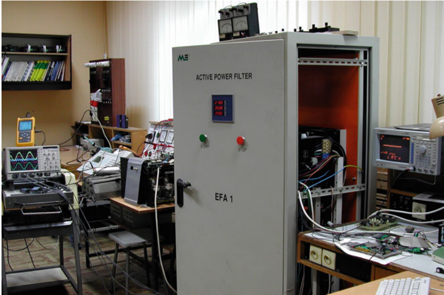
Fig. 5.27 The three-phase shunt APF at the UZ laboratory
