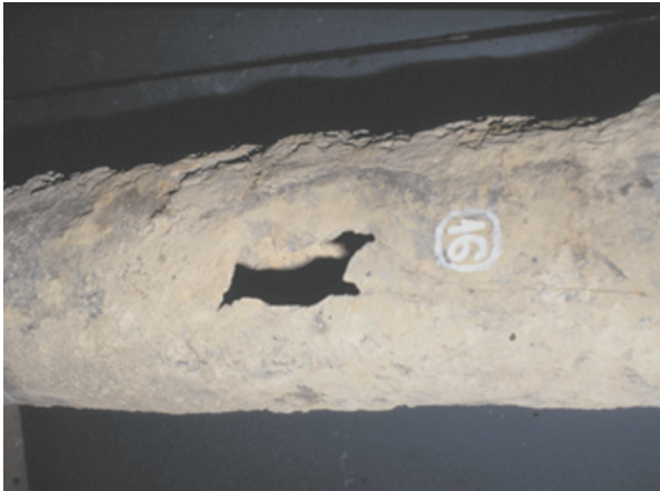
Figure 1. Typical pipeline failure
