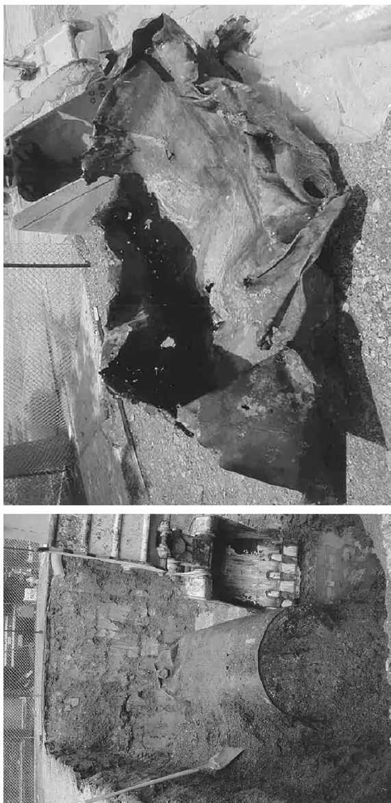
FIGURE 14.1 “Phantom” tanks discovered during site excavations: the leaking fuel oil tank (left) and the remainder of what potentially appeared to be a leaded gasoline tank (right).
