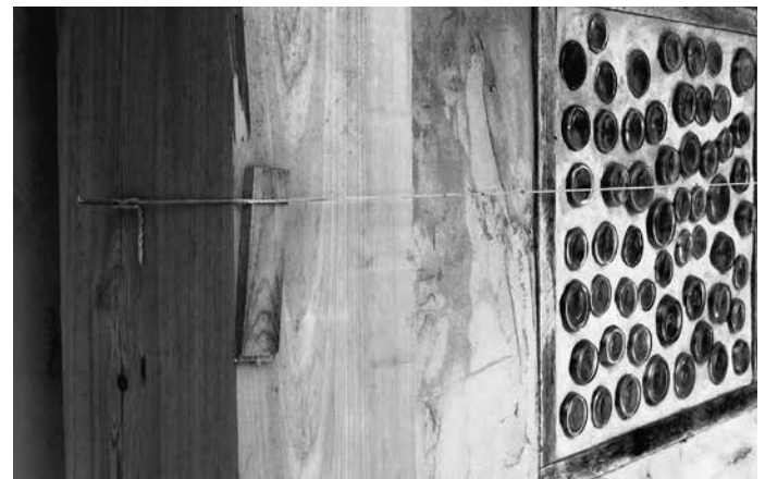
8.17: Mason's clips can be hard to find — and hard to work with if the corner is not perfectly square. You can tack a nylon line onto a post as shown below and hold it proud of the wall with a uniform ( \frac{1}{4} " or \frac{1}{2} " ) wooden shim.
