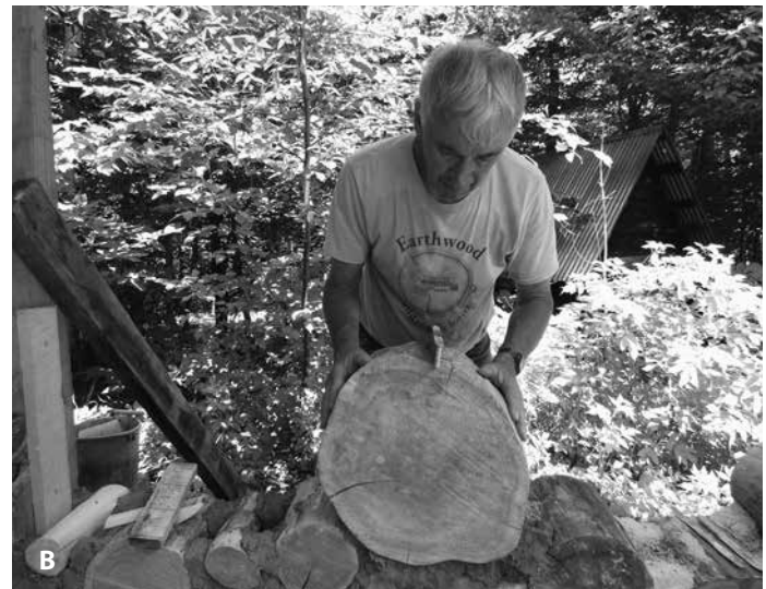
8.14: (A) A large log is a “quality control” opportunity. I check that it is plumb and level, using the plumb bubble of my 4-foot level perpendicular to the run of the wall. (B) A small level across the top is useful, as well.
