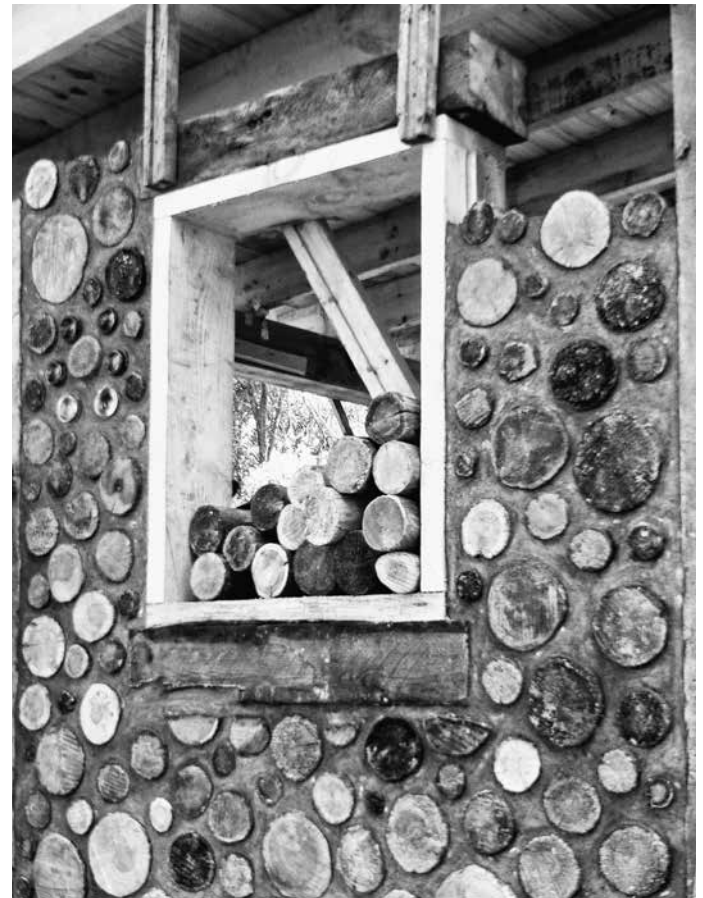
8.24: The bracing to hold the buck vertical is seen clearly. The buck is a good place to store log-ends and mortar pans during construction. Note also the good random rubble placement of log-ends.
