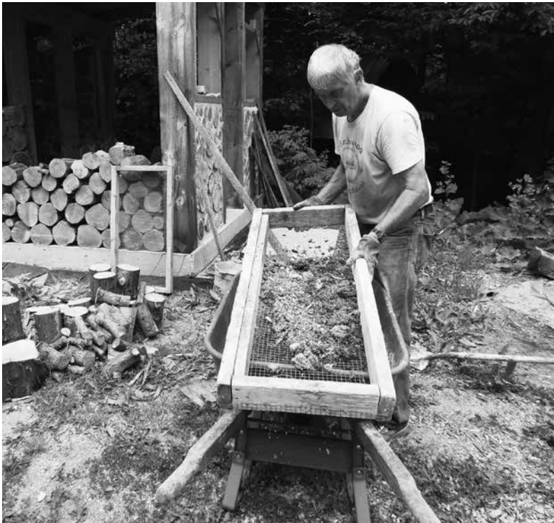
8.5: I shake the sawdust through a half-inch screen, removing various matter that I don't want in my insulation.
