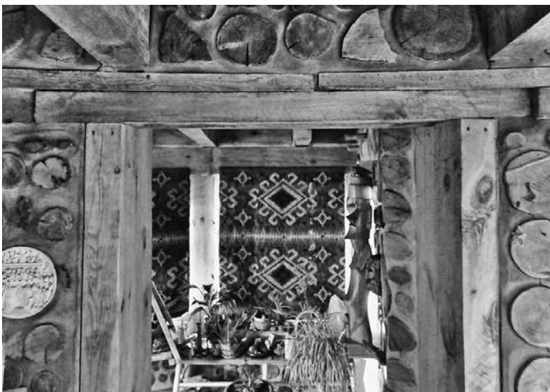
6.16: Top of door frame at Earthwood, made from doubled 4-inch by 8-inch jambs and header.
