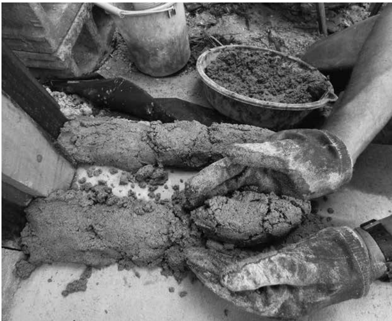
8.7: The two-handed method works well with wider mortar joints, but people with small hands might like it on the 8-inch wall, too. Note the mortar pan in the picture, and the sawdust bucket, both close at hand.
