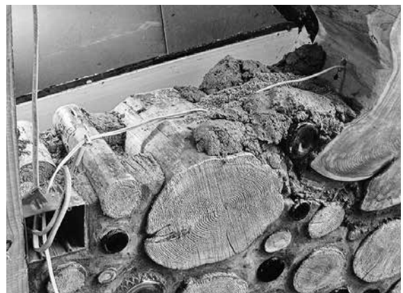
6.28: A double-wide box fastened to a door frame (left side of image) will provide switches for an overhead light, as well as the LED light inside a crystal skull bottle-end feature.
