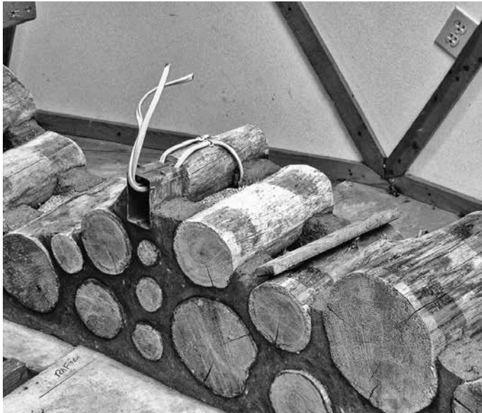
6.25: The wall is built up to and around the electrical box. Notice that plenty of cable is left sticking out of the box to make the connections to the electrical equipment easy for the installer.
