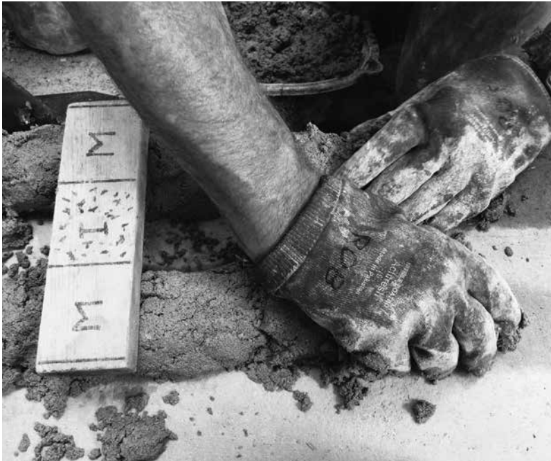
8.6: With the faster single-handed method, my right hand places the mortar on the prepared place for the inner mortar bed, while my left hand does the outer bed. The M-I-M-stick helps me gauge width.
