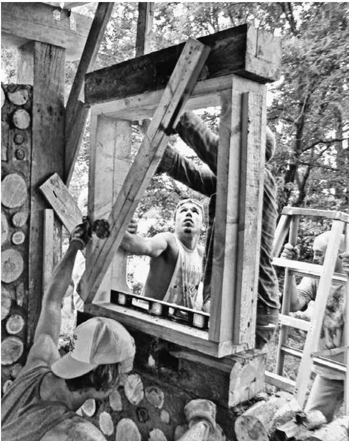
8.23: This window buck is made of full-size 2-by-8 inch lumber. The heavy 6-by-8 inch sill and lintel were an optional design feature which the owner requested. The entire unit was leveled and plumbed, then vertical braces held it plumb against one of the rafters. Note the diagonal brace to hold the buck square, and the key piece on the side.
