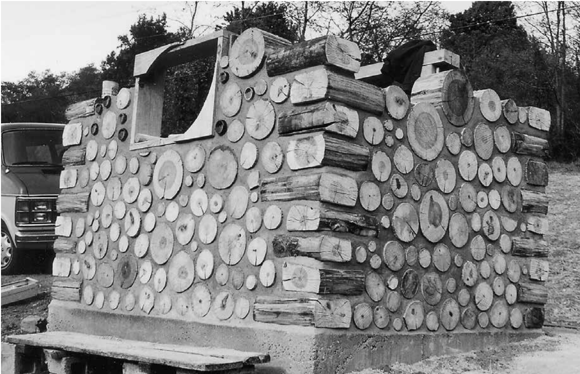
6.10: This small pump-house in North Carolina was made with single-wide quoins, cut from tulip poplar with a chainsaw, then water-sealed to minimize water absorption from mortar to wood. The staggered length of the quoins is clear in this image.
