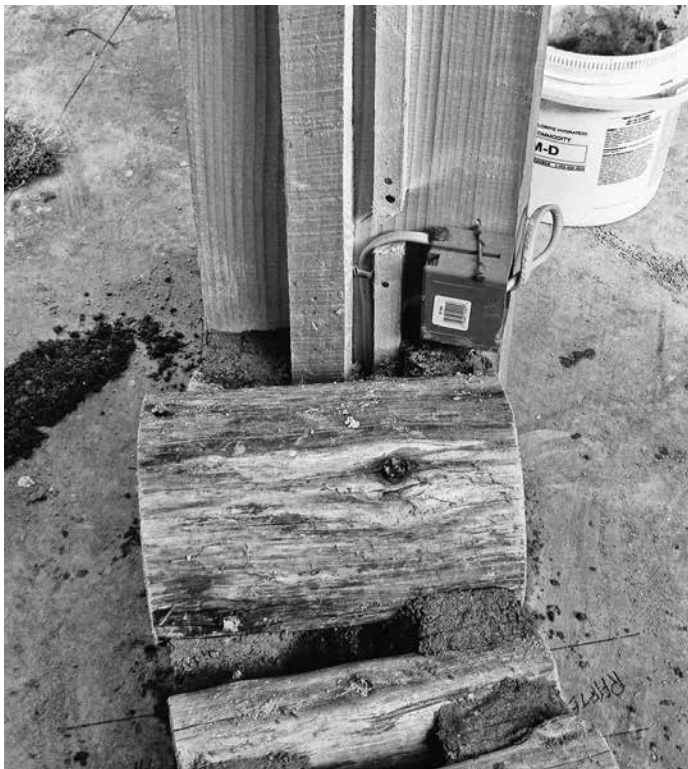
6.27: A view of the other side of the door frame shows the key pieces more clearly, as well as the first course of cordwood masonry.
