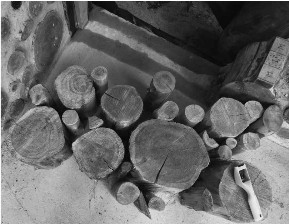
8.1: The area to be worked on this 8-inch cordwood wall (for a sauna) has had a bonding agent applied to the concrete foundation where the cordwood will be laid. A variety of 8-inch log-ends stand within reach.
