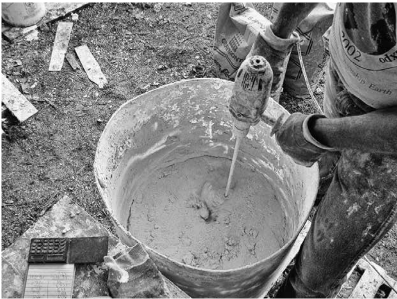
5.13: After measuring the right amounts of lime and water into half of a 55-gallon plastic drum, everything is homogenized with a paddle drill.
