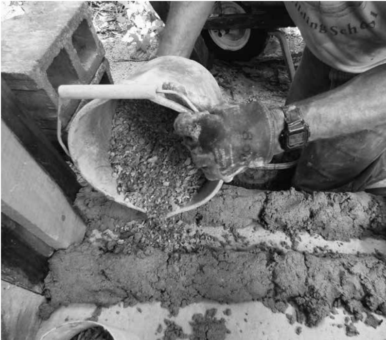
8.8: Pour the insulation between the inner and outer mortar joints with a small spouted bucket, being careful not to spill any on the mortar.
