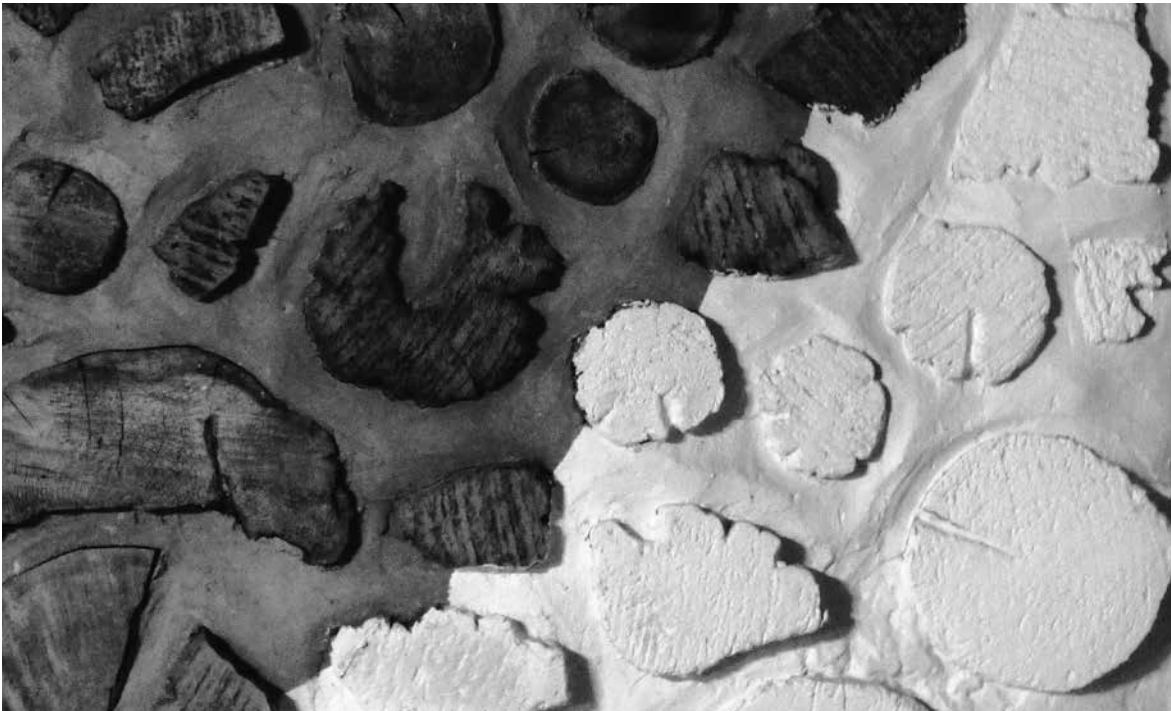
9.16: The texture and relief of the cordwood wall is still evident where the wall is painted.
