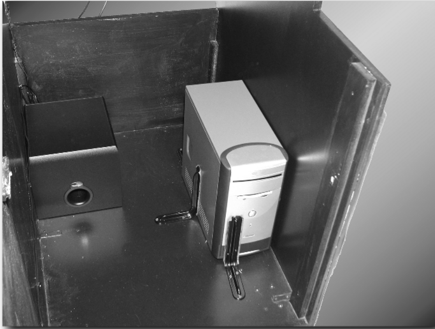
FIGURE 13-11: PC secured in cabinet.
