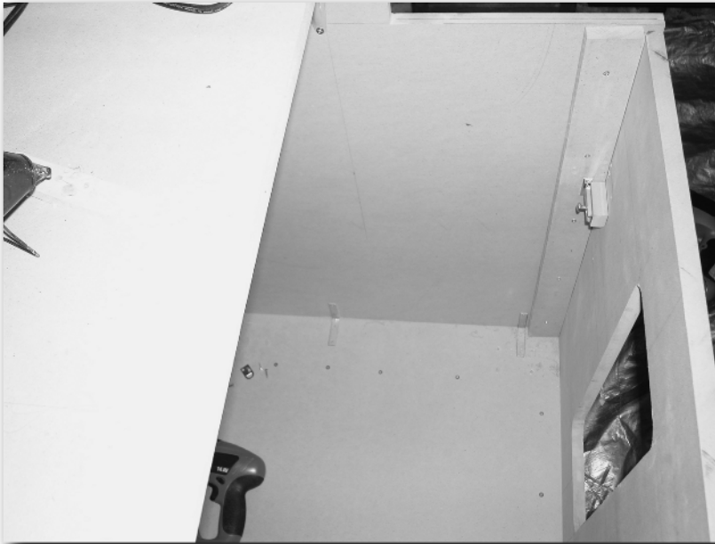
FIGURE 2-25: The cabinet front stop securely mounted to the cabinet side (looking from above).
