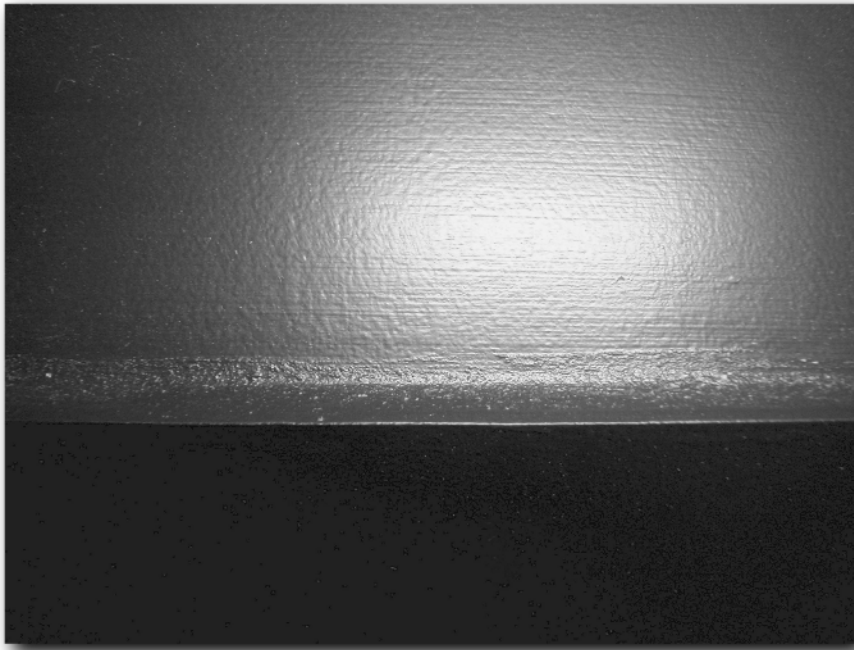
FIGURE 16-1: Close-up of back panels with no visible gaps.
