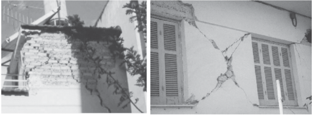
Figure B.24 Shear cracks along the joint bed ( left ) and through the masonry units ( right ) of load-bearing walls observed during the 1999 North Athens (Greece) earthquake
