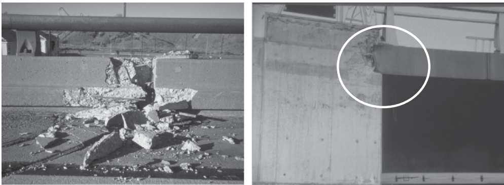
Figure B.44 Pounding damage: between adjacent spans at the Interstate-5 at Santa Clara River in Los Angeles County during the 1994 Northridge (California) earthquake ( left ) and at the abutment of a bridge near Nishinomiya Port in the 1995 Kobe (Japan) earthquake ( right ) ( courtesy of National Information Service for Earthquake Engineering, University of California, Berkeley) Reproduced from: Left: Image: Northridge Collection: NR968 Right: Image: Unknown URL: http://nisee.berkeley.edu/elibrary/
