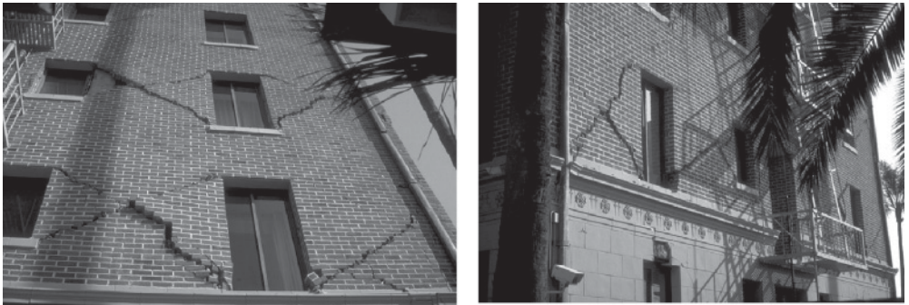
Figure B.11 Diagonal cracks in the infills of an apartment building on Wilshire (Santa Monica, California) in the 1994 Northridge earthquake (courtesy of National Information Service for Earthquake Engineering, University of California, Berkeley) Reproduced from: Left: Image: Northridge Collection: NR158 Right: Image: Northridge Collection: NR156 URL: http://nisee.berkeley.edu/elibrary/
