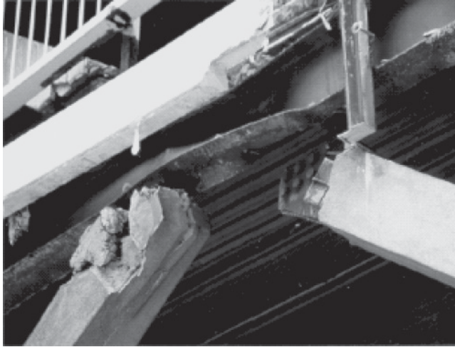
Figure B.34 Local buckling brace-to-beam connection during the 1995 Kobe (Japan) earthquake (after Naeim, 2001)
