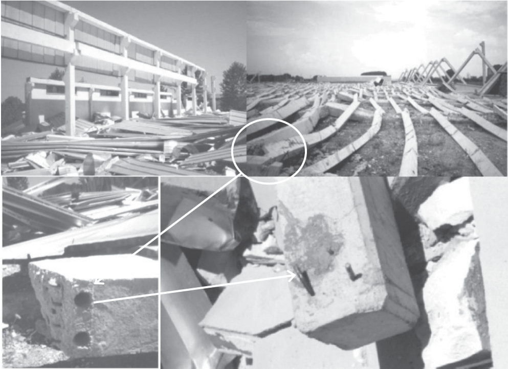
Figure B.16 Collapse of precast RC building during the 1999 Kocaeli (Turkey) earthquake: general damage ( top ) and close-up of the details ( bottom )
