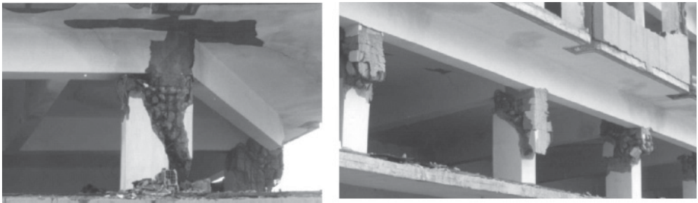
Figure B.4 Shear failures in short columns observed in the 1999 Kocaeli (Turkey) earthquake
