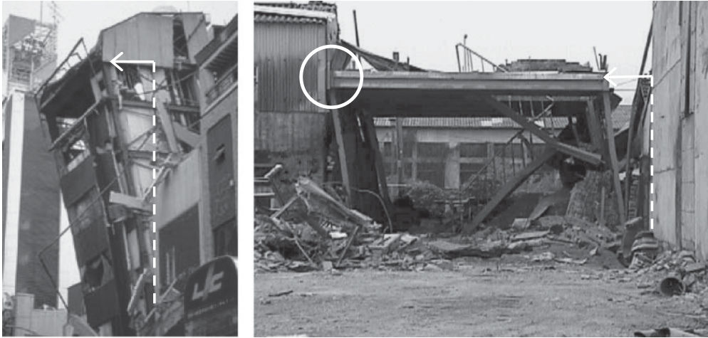
Figure B.37 Excessive lateral displacement during the 1995 Kobe, Japan, (left) and the 1999 Chi-Chi, Taiwan, earthquake (right) (after FEMA, 2000)
