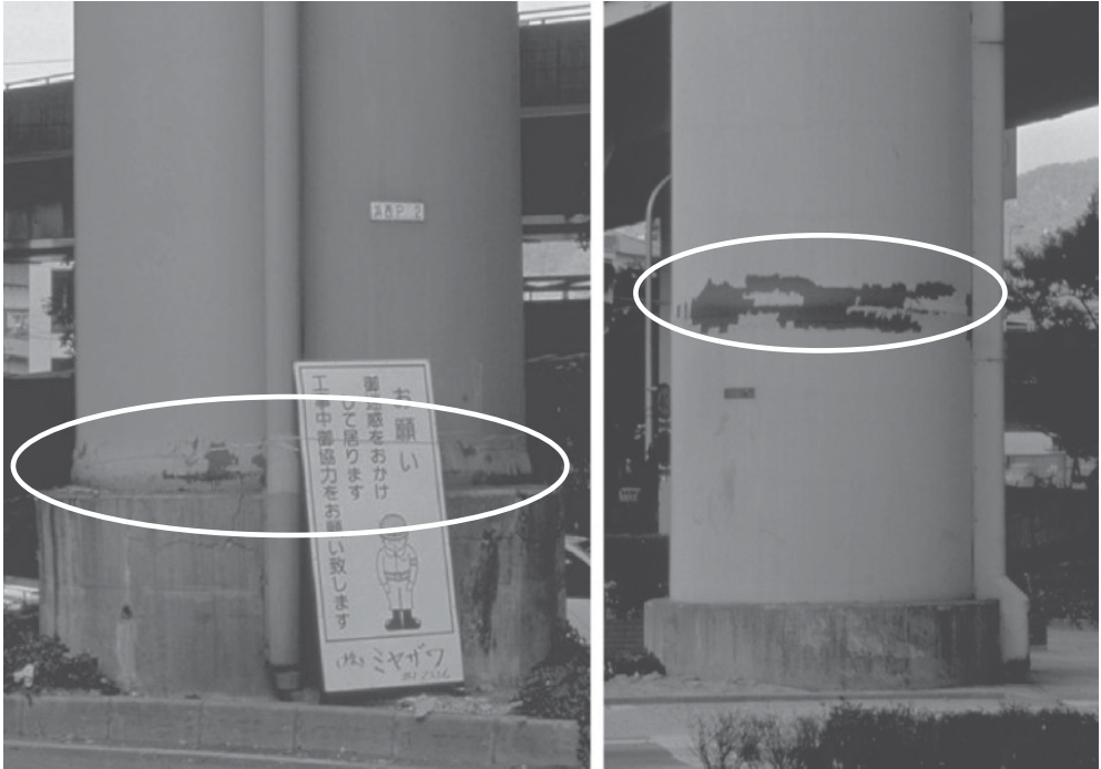
Figure B.51 Elephant foot mode in steel piers of the Collector from Port Island to Kobe during the 1995 Kobe (Japan) earthquake: buckling at the pier base ( left ) and at intermediate height ( right ) ( courtesy of Dr. Matej Fishingier )
