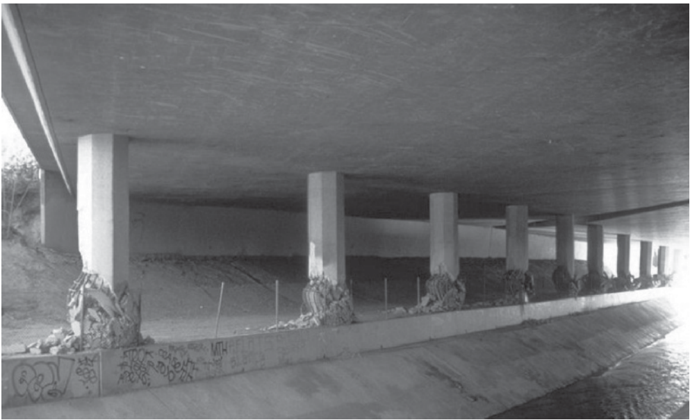
Figure B.47 Flexural plastic hinges in columns connected by a wall, Bull Creek Canyon Channel bridge, 1994 Northridge (California) earthquake ( courtesy of National Information Service for Earthquake Engineering, University of California, Berkeley) Reproduced from: Left: Image: Northridge Collection: NR902 URL: http://nisee.berkeley.edu/elibrary/
