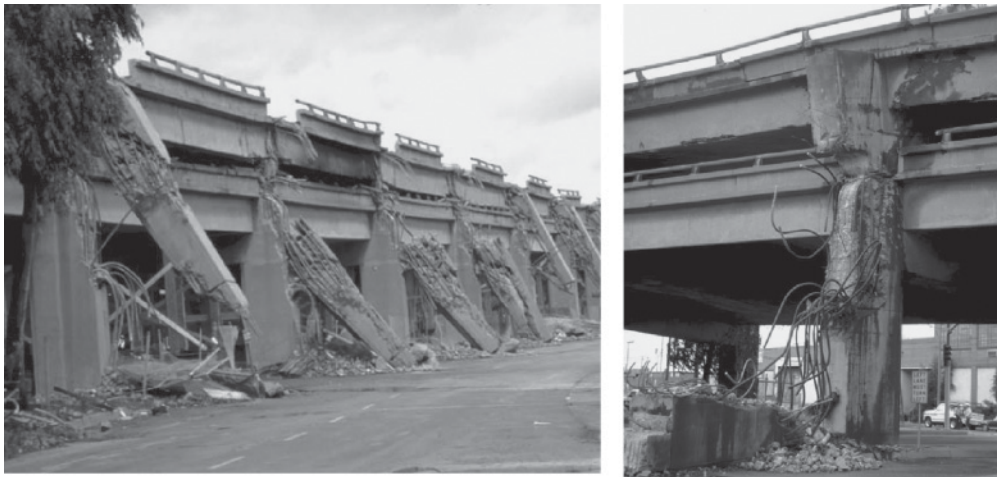
Figure B.55 Sliding shear at top columns of the Cypress Viaduct in the 1989 Loma Prieta (California) earthquake ( courtesy of National Information Service for Earthquake Engineering, University of California, Berkeley) Reproduced from: Left: Image: Karl V. Steinbrugge Collection: S6130 Right: Karl V. Steinbrugge Collection: S6128 URL: http://nisee.berkeley.edu/elibrary/
