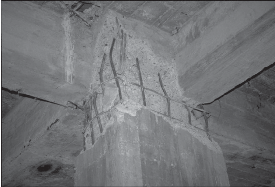
a. Inadequate number of stirrups at the beam-to-column connection
