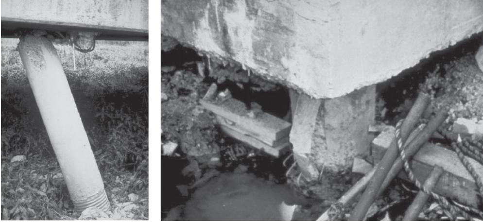
Figure B.56 Failures of piles supporting RC bridges during the 1989 Loma Prieta (California) ( left ) and 1995 Kobe (Japan) ( right ) earthquakes ( courtesy of National Information Service for Earthquake Engineering, University of California, Berkeley) Reproduced from: Left: Image: Karl V. Steinbrugge Collection: S6130 Right: Matej Fischinger – CD ROM URL: http://nisee.berkeley.edu/elibrary/
