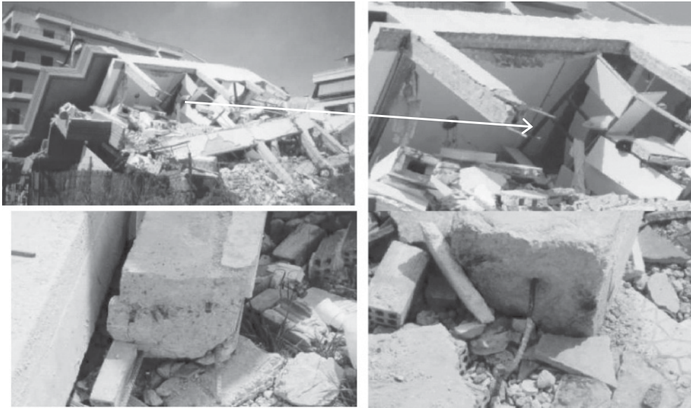
Figure B.19 Collapse of framed structure caused by inadequate anchorage of column longitudinal reinforcement bars in the 1999 North Athens (Greece) earthquake: collapsed frames ( top ) and close-up of the pull-out of the steel bars ( bottom )
