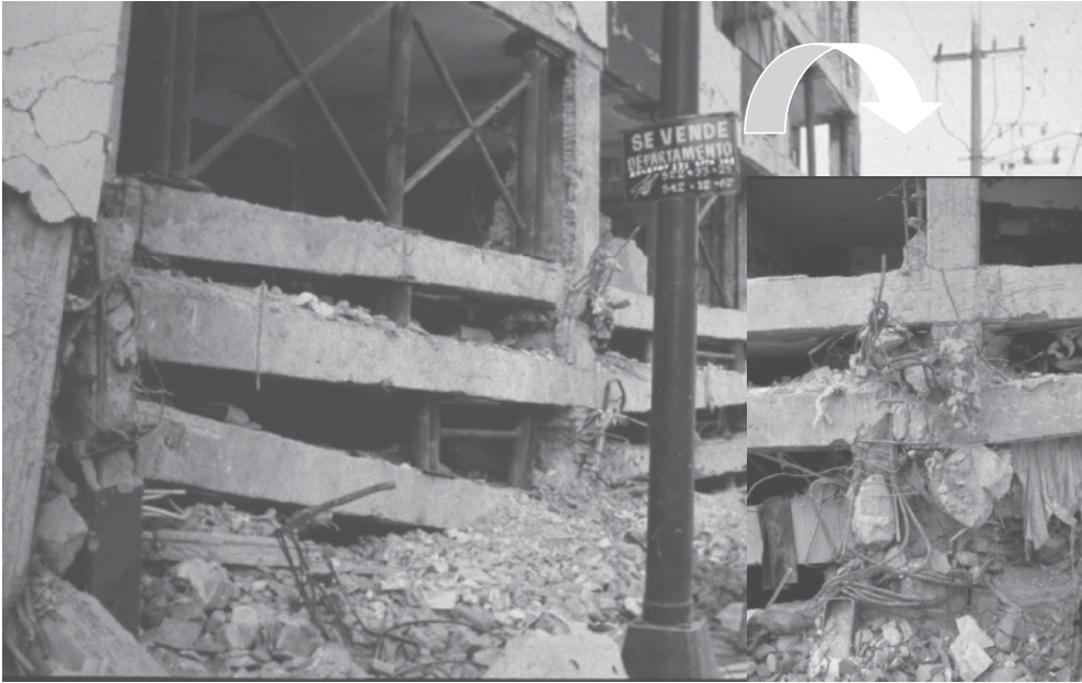
Figure B.13 Soft storeys in multi-storey RC frame caused by resonance in the 1985 Michoacan (Mexico City) earthquake: collapsed frames and inset with close-up of the crushed columns ( courtesy of Dr. Matej Fishingier )
