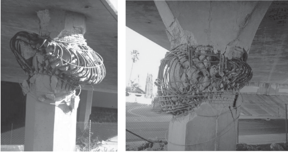
Figure B.46 Confinement failure at a bridge pier top during the 1994 Northridge earthquake ( courtesy of National Information Service for Earthquake Engineering, University of California, Berkeley) Reproduced from: Left: Image: Northridge (California) Collection: NR904 Right: Unknown URL: http://nisee.berkeley.edu/elibrary/
