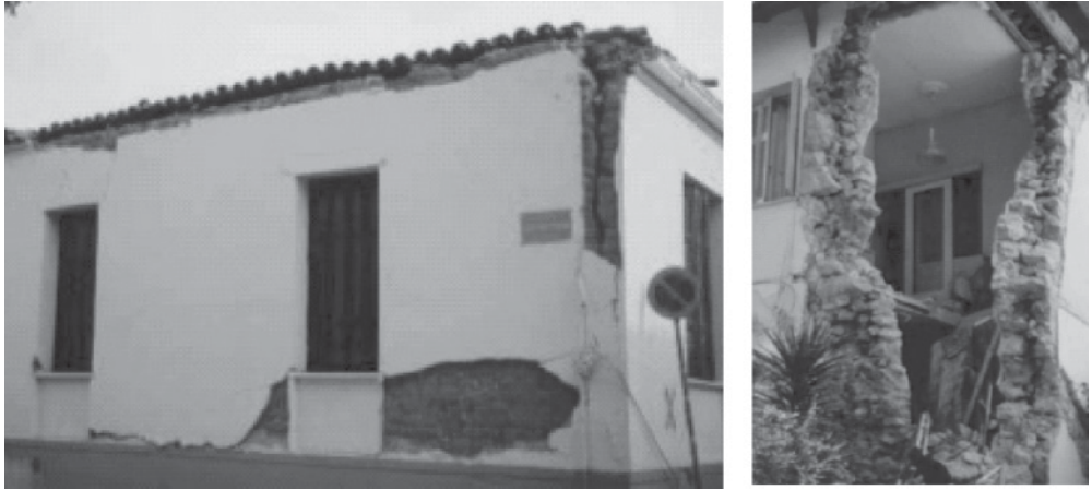
Figure B.26 Corner damage observed during the 1999 North Athens (Greece) earthquake: large vertical separation ( left ) and total collapse ( right )
