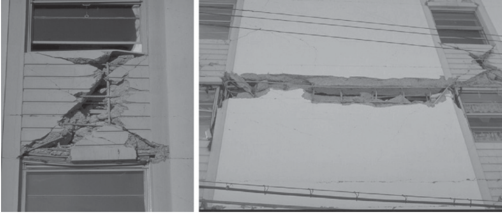
Figure B.22 Typical shear damage ( left ) and cracks at construction joints ( right ) in reinforced concrete slender walls ( courtesy of National Information Service for Earthquake Engineering, University of California, Berkeley ) Reproduced from: Left: Image: Karl V. Steinbrugge Collection: S2073 Right: Image: Karl V. Steinbrugge Collection: S2089 URL: http://nisee.berkeley.edu/elibrary/
