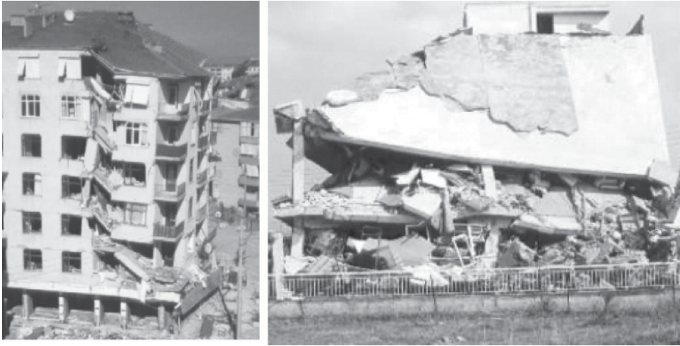
Figure B.14 Collapses caused by torsional effects in RC multi-storey buildings during the 1999 Kocaeli (Turkey) ( left ) and the 1999 North Athens (Greece) earthquakes ( right )
