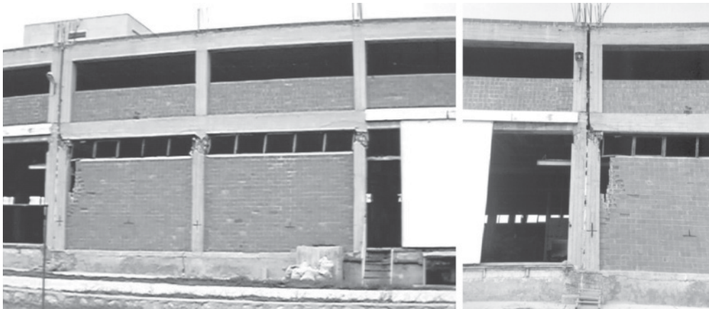
Figure B.7 Shear failures in columns due to interaction with masonry infills in the 1998 Adana–Ceyhan earthquake: short-column effects and shear failure due to the presence of a masonry wall on a single side of the column
