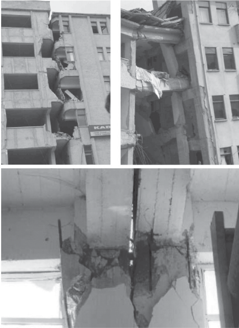
Figure B.17 Severe damage caused by pounding between adjacent buildings with same height ( top-left ), different height ( top-right ) in the 1999 Kocaeli (Turkey) earthquake and close-up of damage due to hammering between adjacent columns ( bottom ) in the 1999 North Athens (Greece) earthquake
