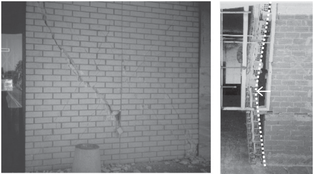
Figure B.27 Damage observed in non-structural walls of unreinforced masonry buildings: cracks along joint beds and through the masonry units in the brick facade of the Broadway Store in the 1994 Northridge (California) earthquake ( left ) and global buckling of slender brick wall in a private house during the 1999 North Athens (Greece) earthquake ( right ) ( courtesy of National Information Service for Earthquake Engineering, University of California, Berkeley) Reproduced from: Left: Image: Karl V. Steinbrugge Collection: S2073 URL: http://nisee.berkeley.edu/elibrary/
