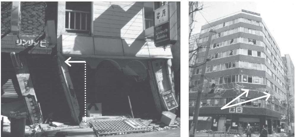
Figure B.12 Soft storeys in RC structures in the 1995 Kobe (Japan) earthquake: collapse of the first (left) and intermediate (right) storey (courtesy of Dr. Matej Fischinger) Reproduced from Matej Fischinger – CD ROM, with permission.
