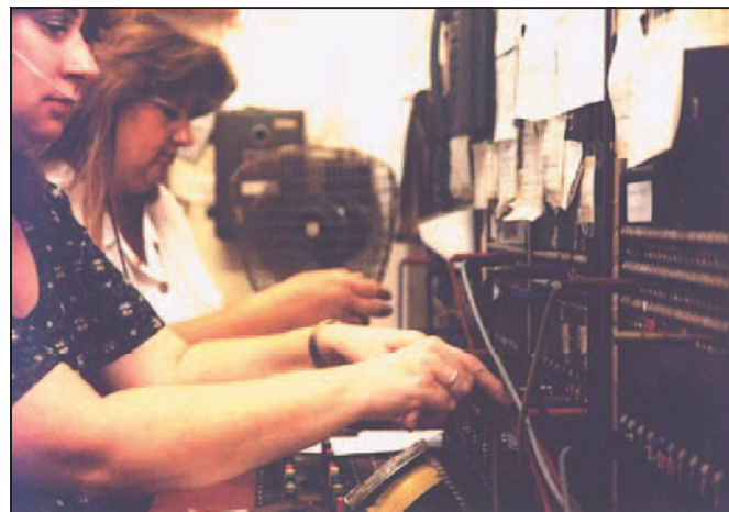
A hospital switchboard in 1995—shows the operators' directory and temporary notes. With permission from Martin Loach
