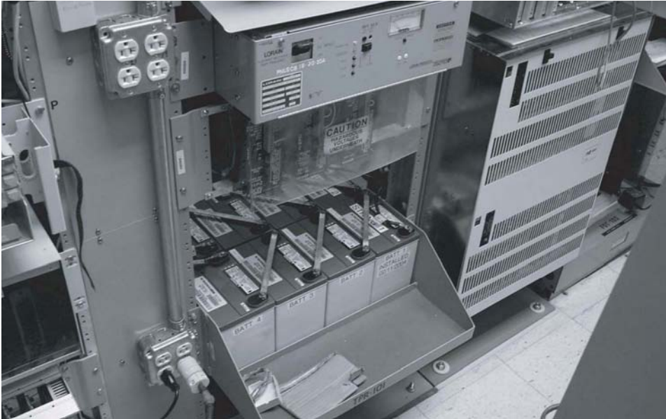
Fig. 4.11 Small 6-cell VRLA monoblocs on a frame-mounted tray (four monoblocs visible in front and four in back in middle-bottom of picture). (Photo courtesy of M.W. Migliaro.)
