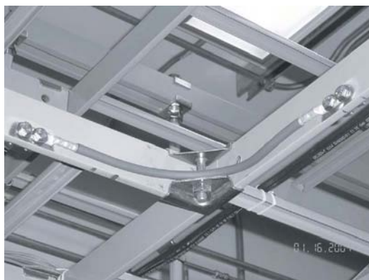
Fig. 5.77 Cable rack bonding. Note the paint has been removed where the bonding strap connector lugs are fastened to the cable rack stringers.
