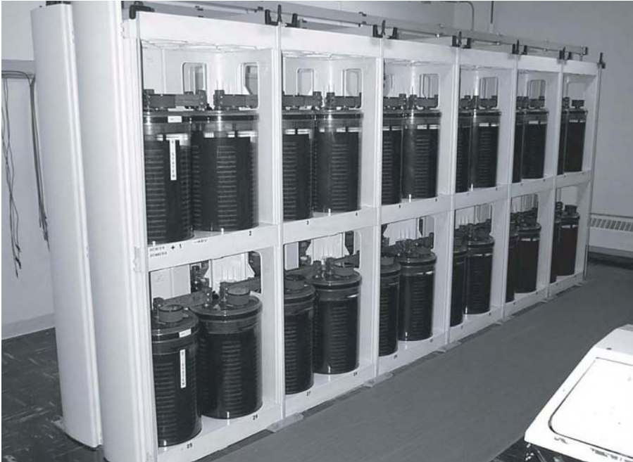
Fig. 4.12 Battery consisting of round cells and seismic zone 4 rack installed in southeastern Alaska. Round cells are not very space efficient, but they have a relatively long life when properly operated and maintained.
