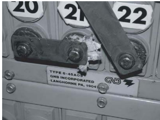
Fig. 6.52 Post seal leak on cell 21 of a VRLA battery. (Photo courtesy of M.W. Migliaro.)
