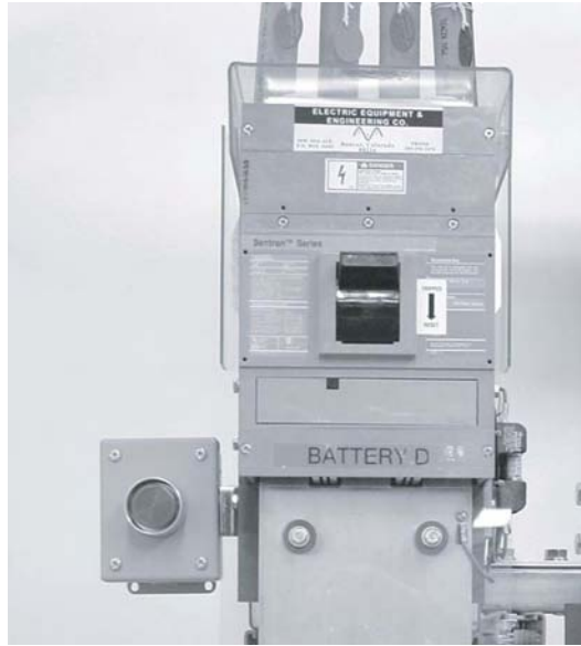
Fig. 3.47 Trip control (red push-button on lower left is shown for illustration only as a trip control serves no useful purpose located so close to the disconnect switch or circuit breaker). (Photo courtesy of Electric Equipment & Engineering Company).
