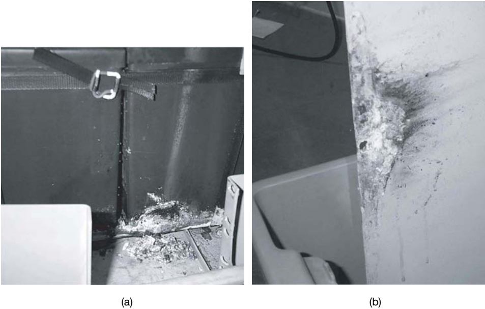
Fig. 4.23 Leaking cell at customer premises—the cell cracked due to shipping or installation handling, allowing electrolyte to leak onto the grounded metal battery enclosure. Since electrolyte allows current flow, the resulting short circuit generated enough heat to burn a hole through the battery jar (a) about 1 in. across and enclosure (b) about \frac{3}{8} in. across like a blowtorch.
