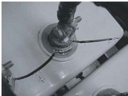
Fig. 6.38 Cracked cell cover caused by corrosion in the post seal. (Photo courtesy M.W. Migliaro.)
