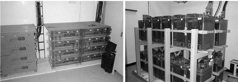
Fig. 1.13 Battery systems (24-cell VRLA on the left and 24-cell VLA on the right).
