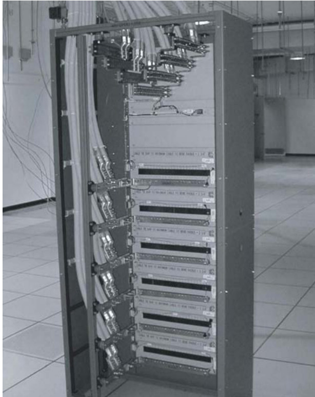
Fig. 5.27 Secondary distribution bay. The return busbars are at the top and the individual distribution busbars for each circuit breaker panel are below (the panels shown are empty). (Photo courtesy of Schultz Brothers Electric Company.)
