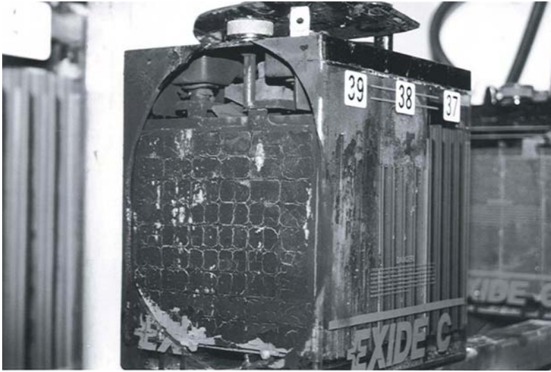
Fig. 6.53 Cell explosion in UPS battery. (Photo and description courtesy of M.W. Migliaro.)
