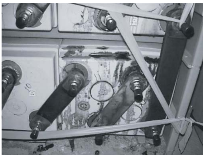
Fig. 6.61 VRLA Thermal runaway. (Photo courtesy of M.W. Migliaro.)
