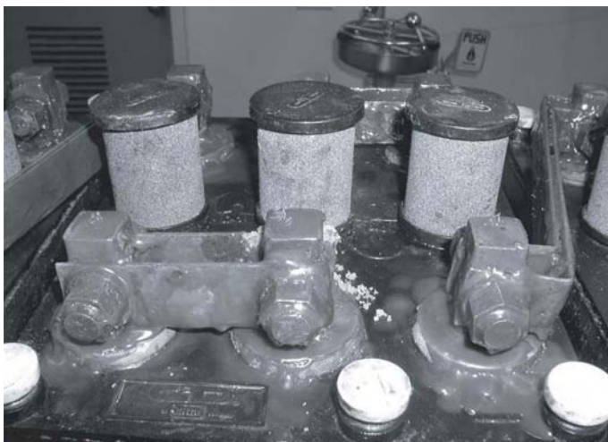
Fig. 6.57 Excessive oxidation inhibitor compound. (Photo courtesy of M.W. Migliaro.)
