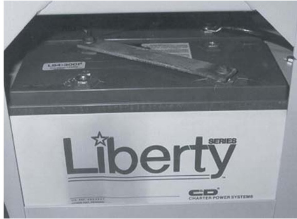
Fig. 4.25 Heat damage to a 2-cell VRLA monobloc from thermal runaway—note discoloration in the area of the letters “Lib.” (Photo courtesy of M.W. Migliaro.)
