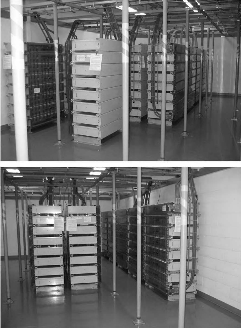
Fig. 1.21 Redundant VRLA battery installation ( upper , B-Blue; lower , A-Red). (Photos courtesy of Nick Nichols.)
