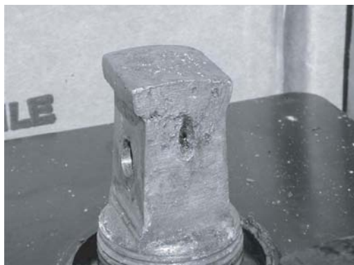
Fig. 6.37 Battery post deformation caused by fastener overtorque. Note that the battery post is deformed in the shape of an anvil (and is called “anvilng”). (Photo courtesy M.W. Migliaro.)
