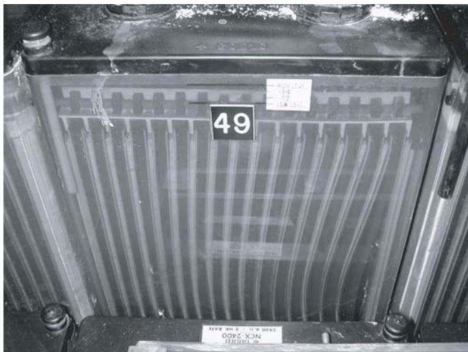
Fig. 6.59 Plate bowing in cell in 19-year-old battery. (Photo and description courtesy of M.W. Migliaro.)
