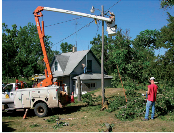
FIGURE 6–7 Crews of specialists repair electrical transmission lines damaged during a tornado in 2004. (Photo courtesy of David Lawrence, Cindy Fay, and Rick Ewald, NOAA, 2004)
