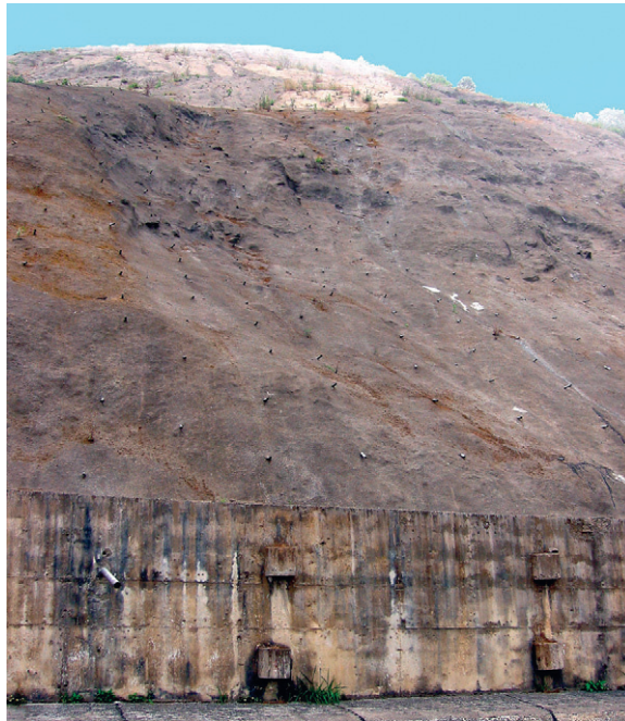
FIGURE 4-5 Slope covered with concrete and outfitted with drainage pipes to prevent landslides.
