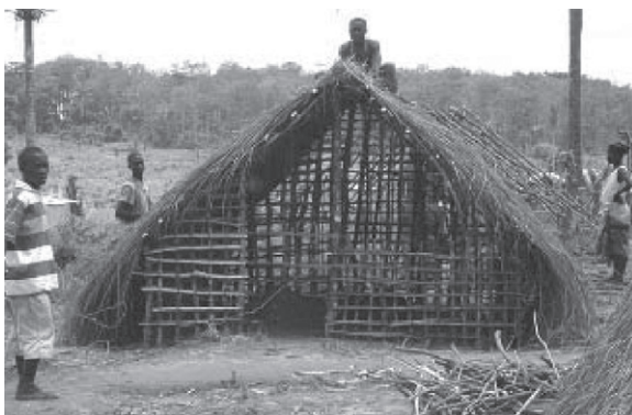
FIGURE 6–5 Shelters being constructed by displaced persons in a camp in Liberia, 2001. (Photo courtesy of Fiona Shanks, USAID/OFDA)
