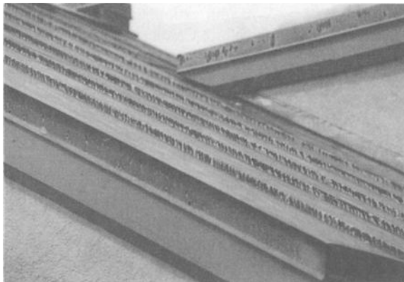
Figure 5 – Discoloration found largely on standing seams and trim on coastal building roof after approximately nine years.
