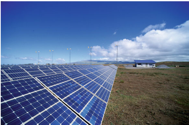
Fig. 6.6 Photovoltaic panels (this photograph is from SunPower, NREL 13823)
