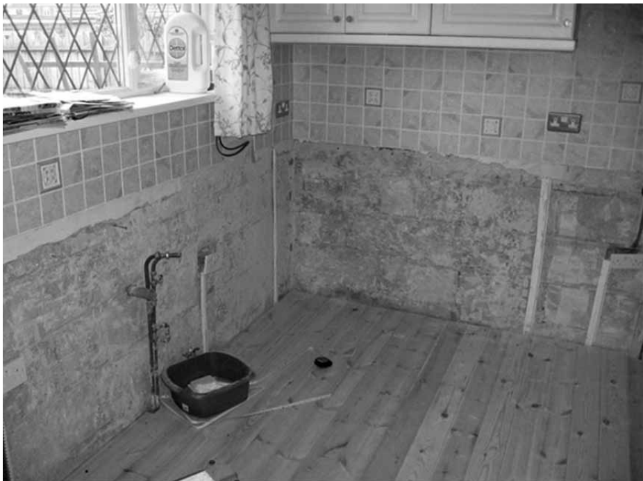
Figure 7.1 An example of the 'stripping out' process endured by many residents in Hull after the 2007 flood: Where the affected property has been stripped back to its bare structure in order to facilitate repair
