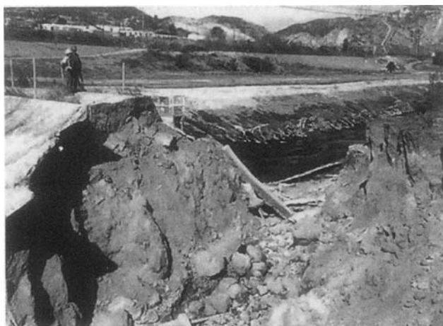
Figure 21. Power plant tailrace dike failure following the 1994 Northridge Earthquake.
