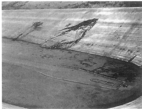
Figure 31. 1956 rapid drawdown landslide in the Upper Stone Canyon Reservoir.
