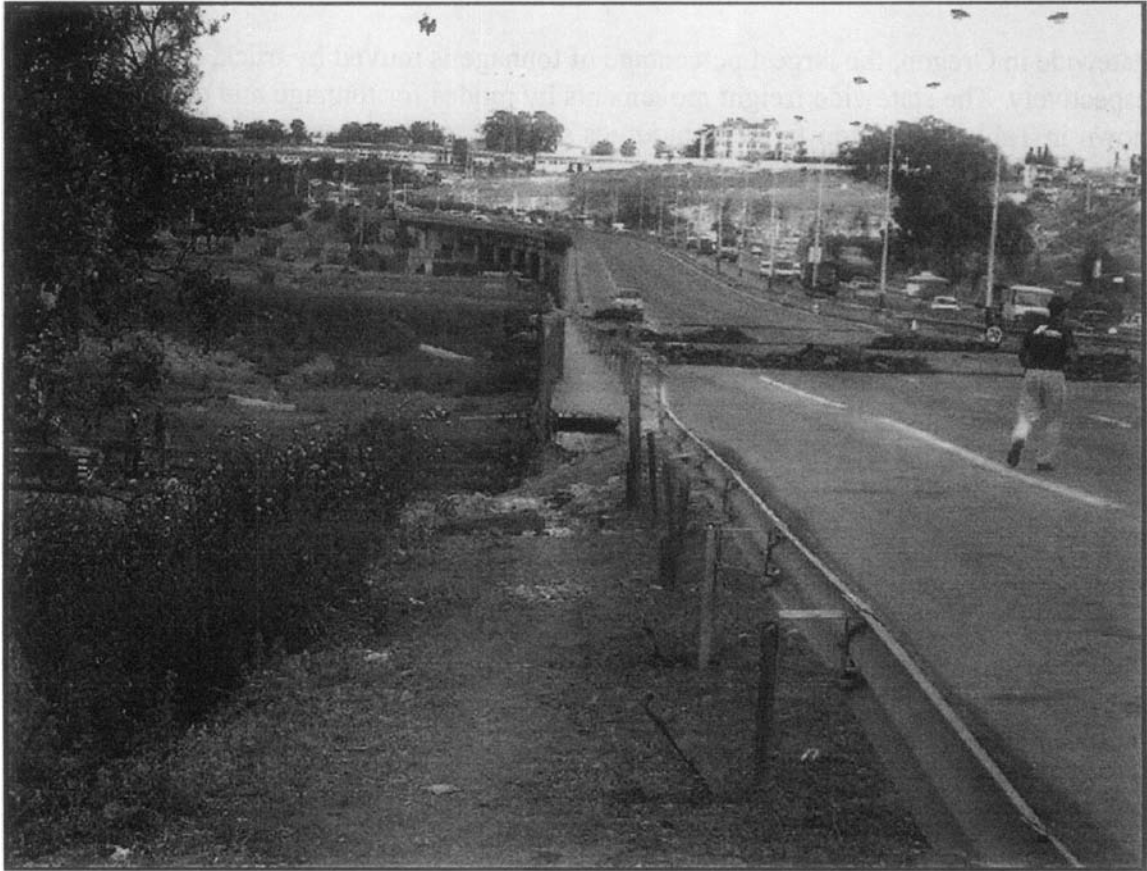
Figure 3. One of two parallel bridges failed in the 2003 Zemmouri, Algeria earthquake causing traffic to be rerouted to the undamaged bridge (Photo credit: Mark Yashinsky).
