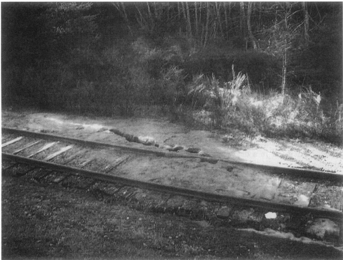
Figure 2. Damage to railway from liquefaction in the 2001 Nisqually, Washington earthquake (photo credit: William Byers).
