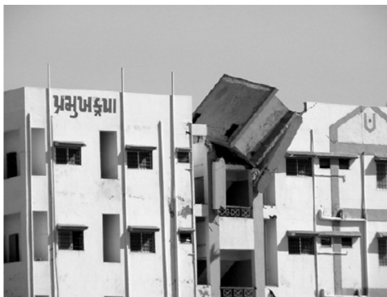
Fig. 11.8 Failure of water tank over the top of a multistorey building (Photo by Jaswant N. Arlekar)
