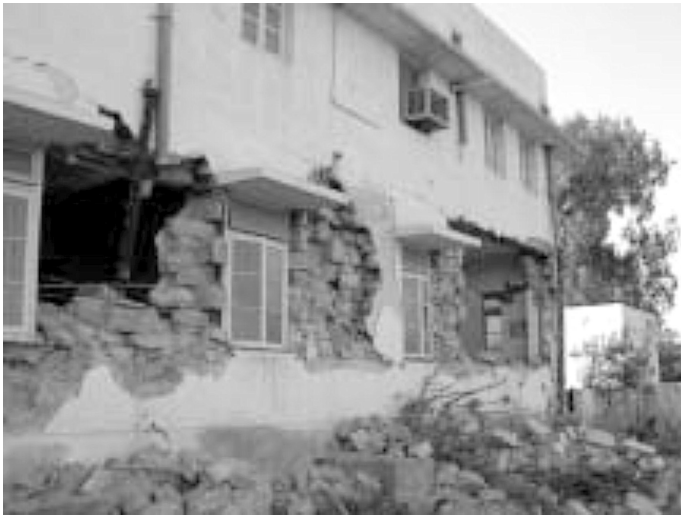
Fig. 11.4 Failure of a typical stone masonry building
