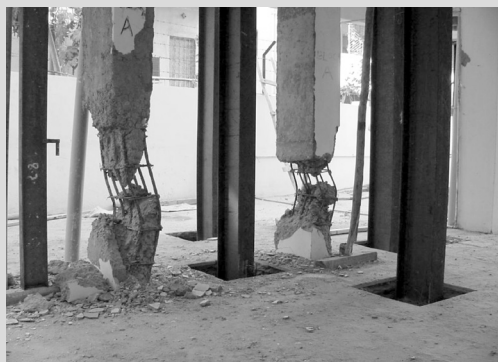
Fig. 11.5 Column failures due to non-ductile detailing
