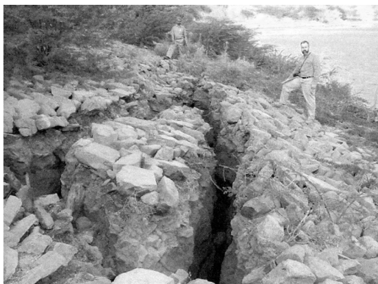
Fig. 11.3 Failure on upstream face of earthen dam
