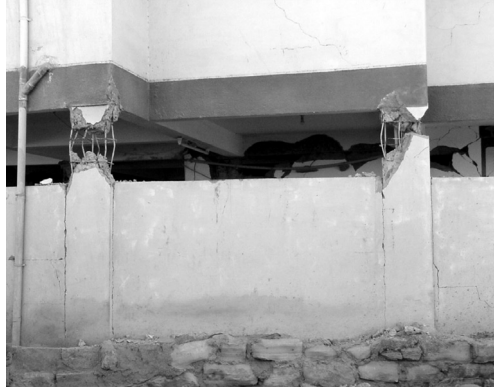
Fig. 11.7 Poorly compacted concrete due to congestion of reinforcement at the top of columns
